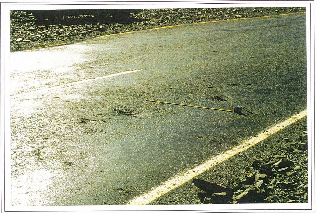
Figure 3.10 Rockfall impact marks at Site 4. Inside lane closest to cut batter is in foreground.
