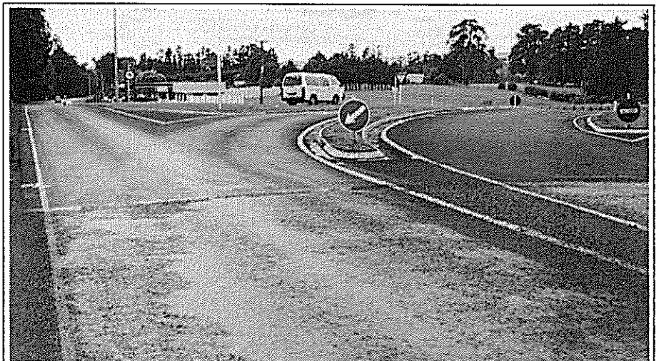
Figure 6.6 Trial site at intersection of SH22 and Glenbrook-Waiuku road, showing transport of flushed bitumen onto the OGEM.
