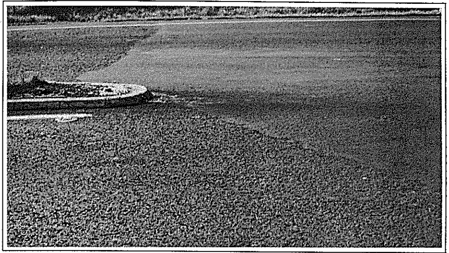
Figure 6.3 Mix 2 Slag OGEM pavement on SH22 lanes shows fretting, as compared with the fine Mix 2/3 Slag at the intersection.
