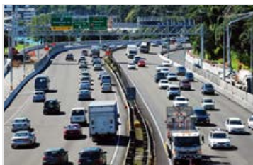
Auckland's Victoria Park Tunnel, barriers on either side completed at St Marys Bay. (JPG, 106KB)
