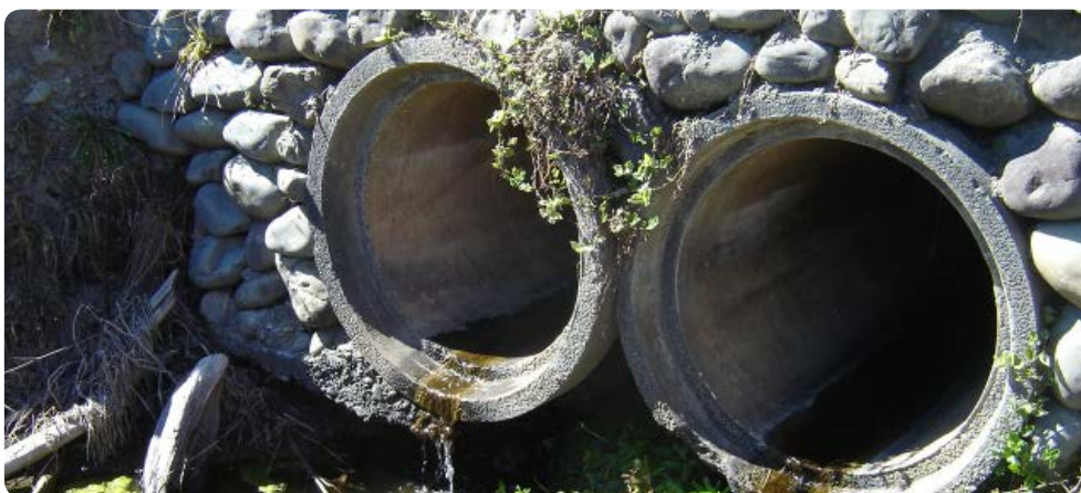
FIGURE 4 Rock armoured on the wall behind these culverts reduces erosion, however retrofit is required to ensure the culverts are not perched
