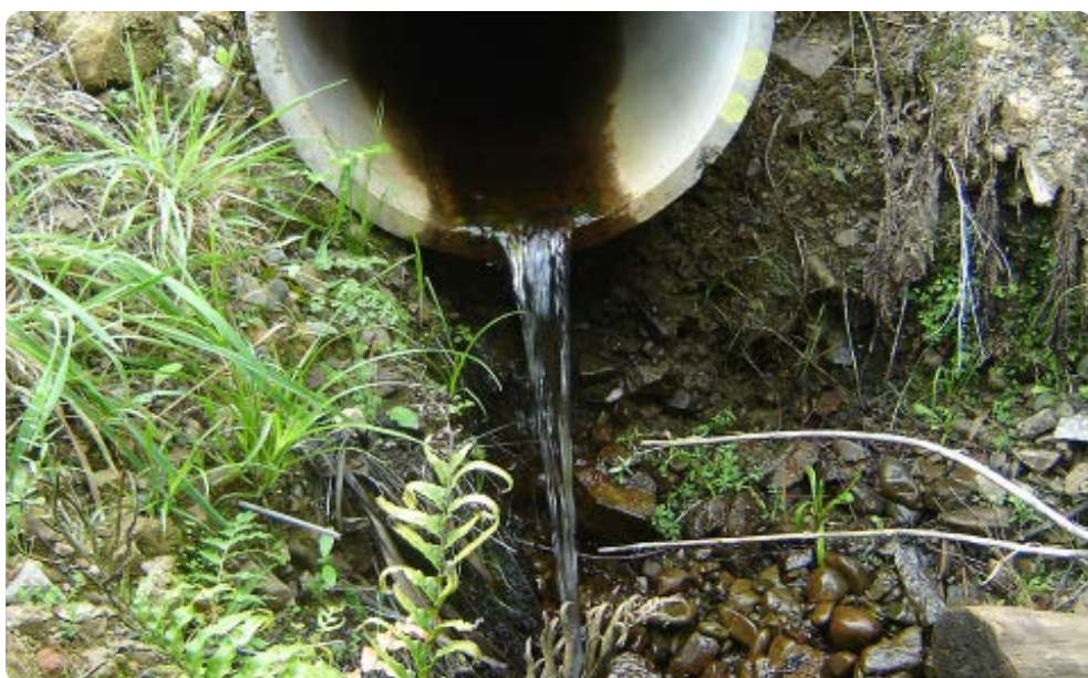
FIGURE 5 Perched projected culvert presents a complete fish passage barrier to upstream migrants
