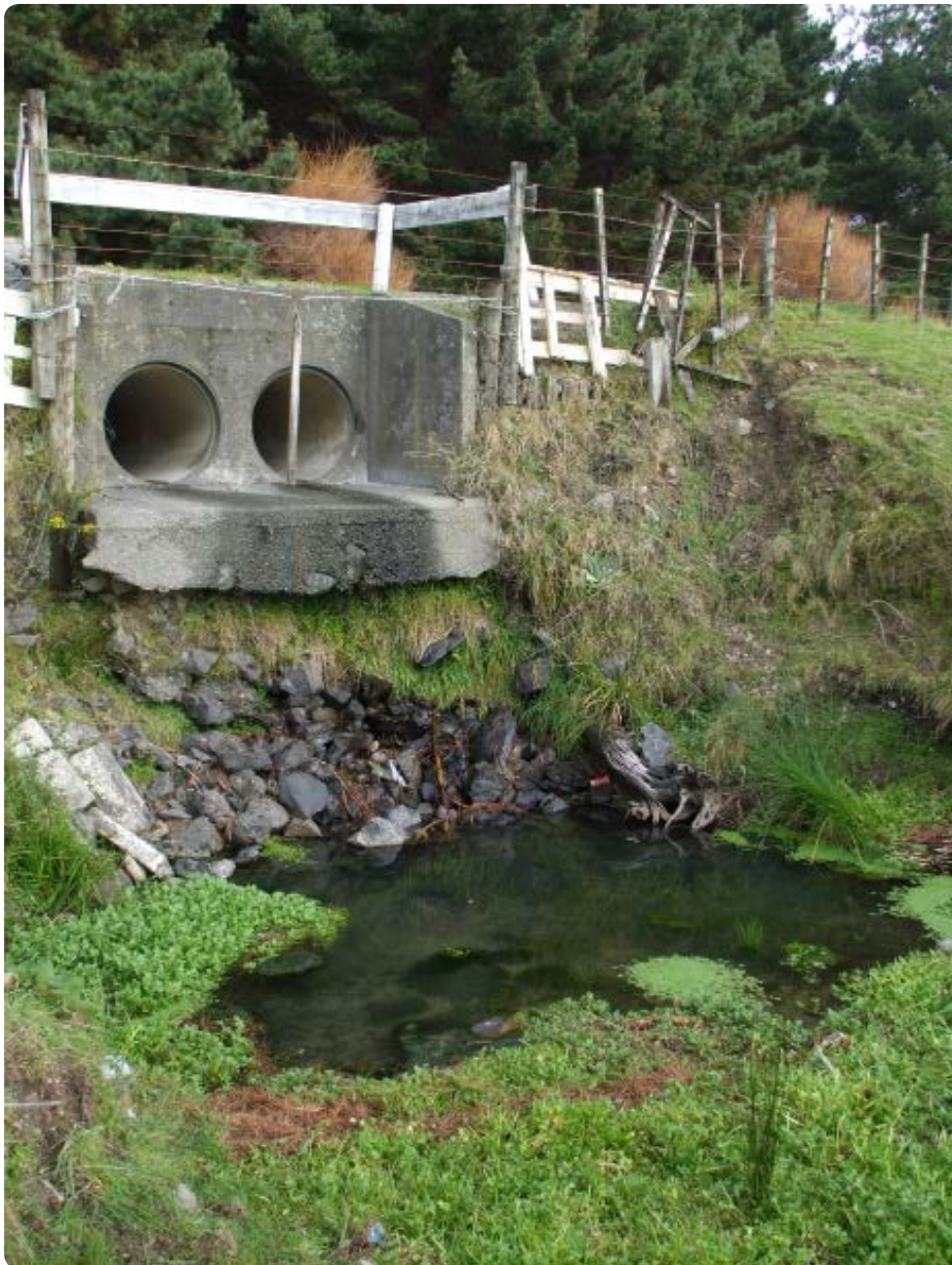
FIGURE 2 An example of a perched culvert - this is not what the NZTA seeks
