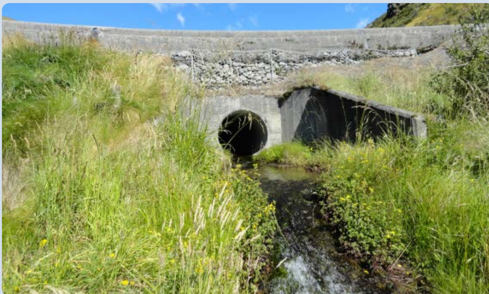
FIGURE 6 The culvert in Coach Stream where it is beneficial to prevent fish passage for the protection of native fish populations from trout
