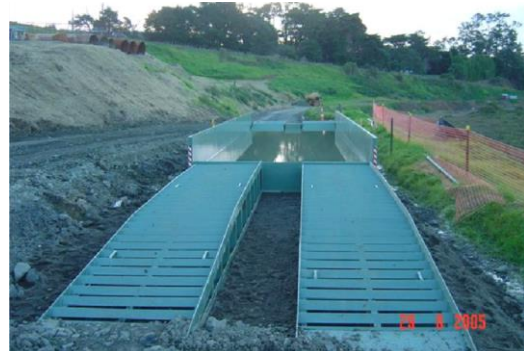
Example of Truck Wash & Shaker Ramp
