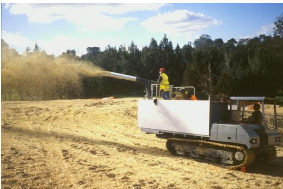
Straw mulch being blown onto a state highway project to reduce erosion
