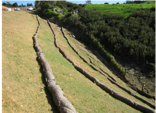
Filter Socks used for slope flow diversion (image provided by Erosion Control Co. Ltd.)
