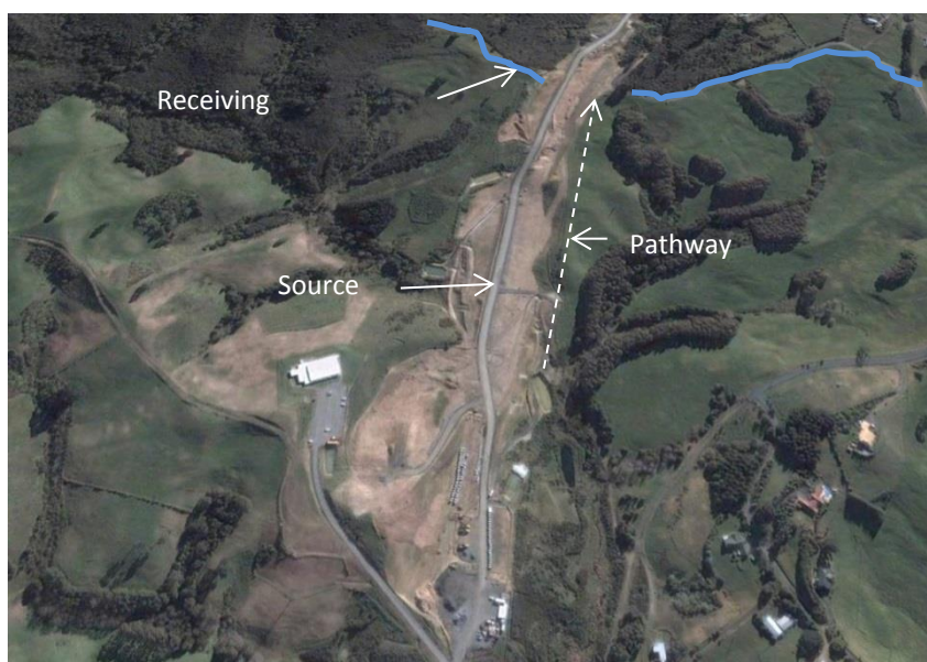
State highway construction showing earthwork area and limited pathways prior to entry into streams
