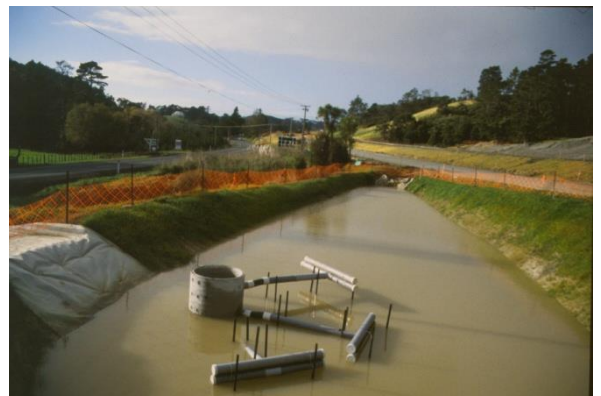
Sediment retention pond to capture state highway sediments
