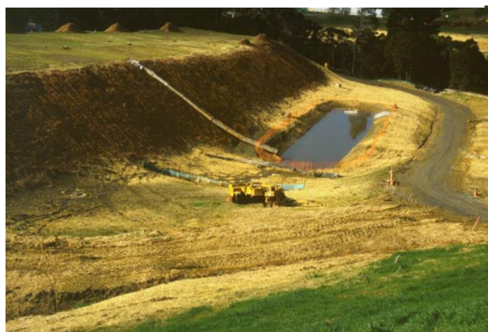
Flume conveying dirty water into sediment retention pond
