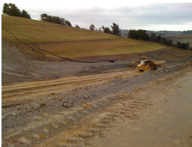
Contour drains established on embankment as a water control measure in conjunction with progressive stabilisation. Note novacoils directing flow down to lower stabilised slope.
