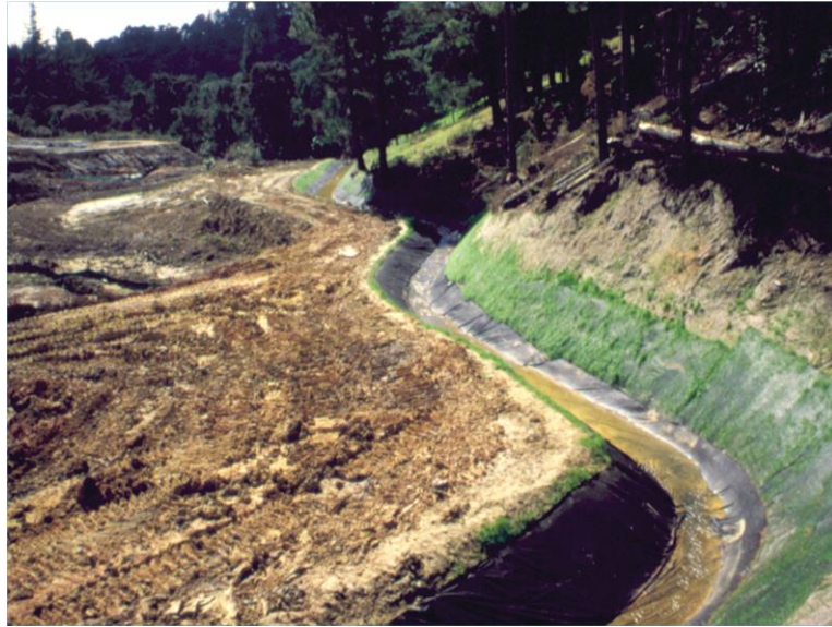
Cleanwater diversion used to isolate upper cleanwater flows from the works area.
