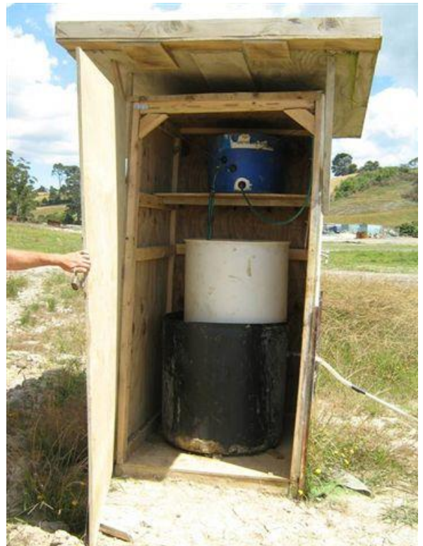
Rain Activated Flocculent Dosing
