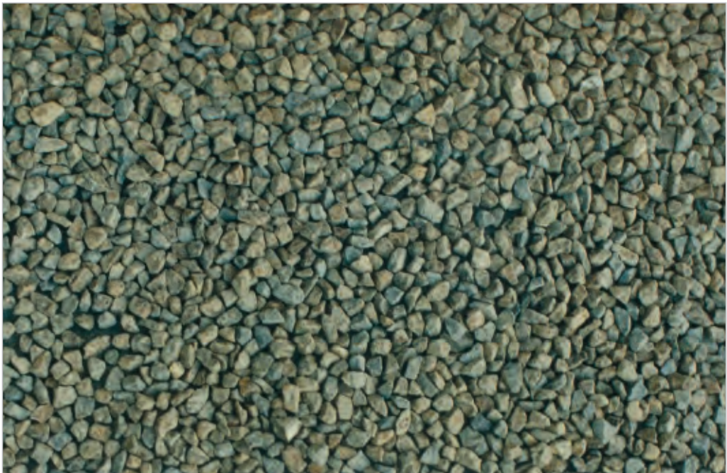
Figure 11-3 Previously advice was to aim for a chip spread-target rate as shown at the top of this page. This is now considered as over-chipping. The image at the bottom of the page shows a very over-chipped seal.
