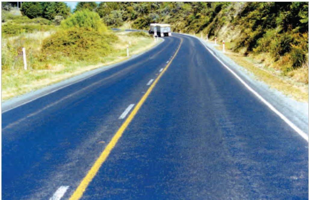
Figure 3-35 This road shows a slick, bleeding or flushed surface that has low friction and therefore low skid resistance. Photo courtesy of Mark Owen, Transit NZ
