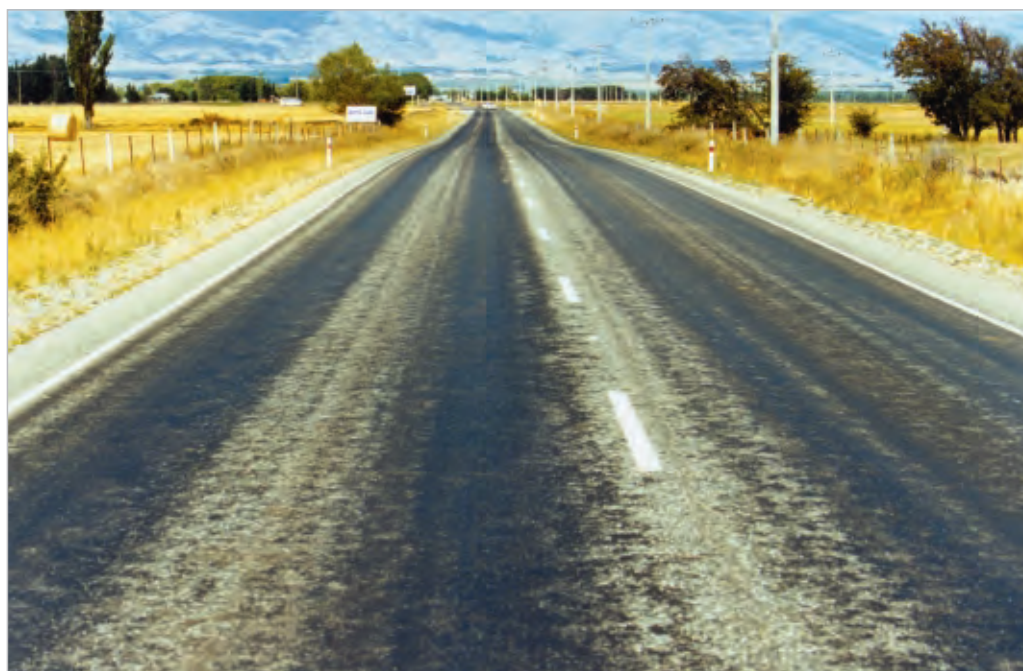
Figure 7-8 A surface in which the wheelpaths have flushed. Note evidence of vapour venting (many small circles of bitumen) on the surface. Photo courtesy of Mark Owen, Transit NZ
