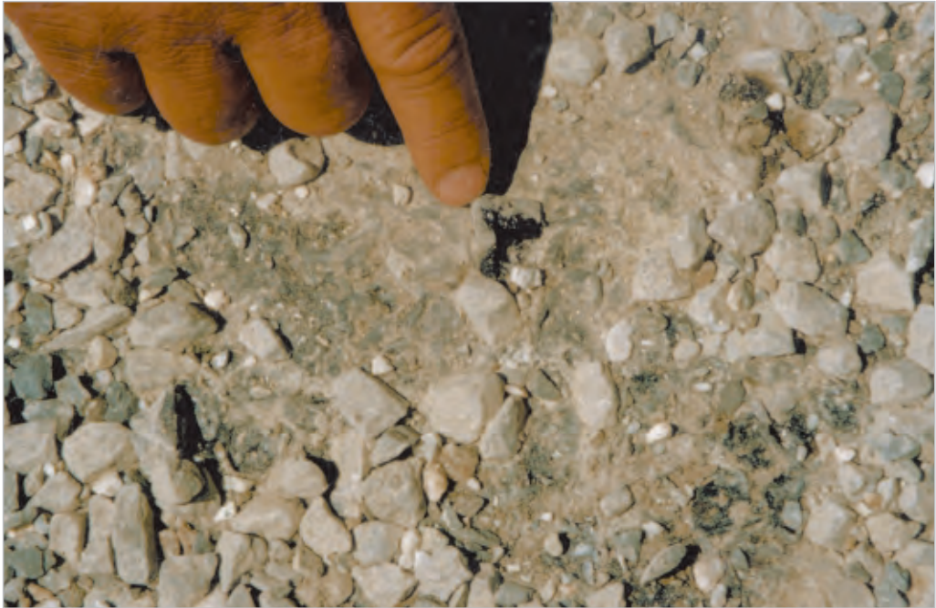
Figure 12-4 Chip loss caused by dirty chip in the seal.
