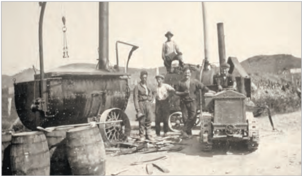
Figure 1-3 This bitumen heating kettle (left) being used in Taranaki was the way to heat bitumen in the 1920s. The fire, stoked with staves from empty bitumen barrels, was in the firebox under the kettle. The firebox gases passed around all sides of the kettle. Photo courtesy of John Matthews, Technix Group Ltd
