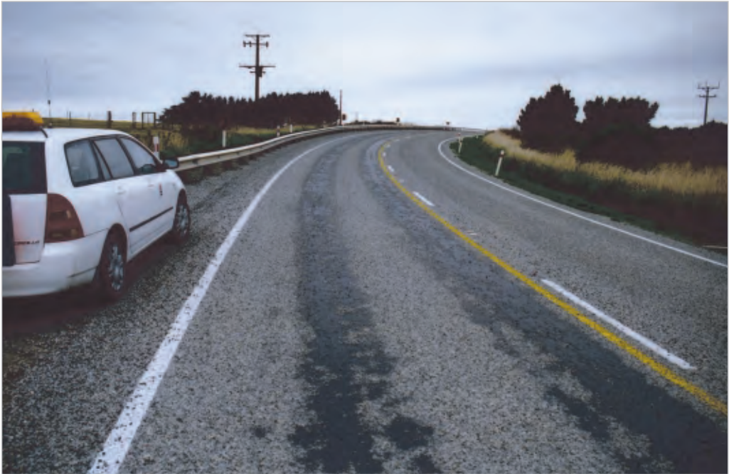
Figure 12-5 Chip loss can occur within 48 hours after chipsealing. Photo courtesy of Les McKenzie, Opus
