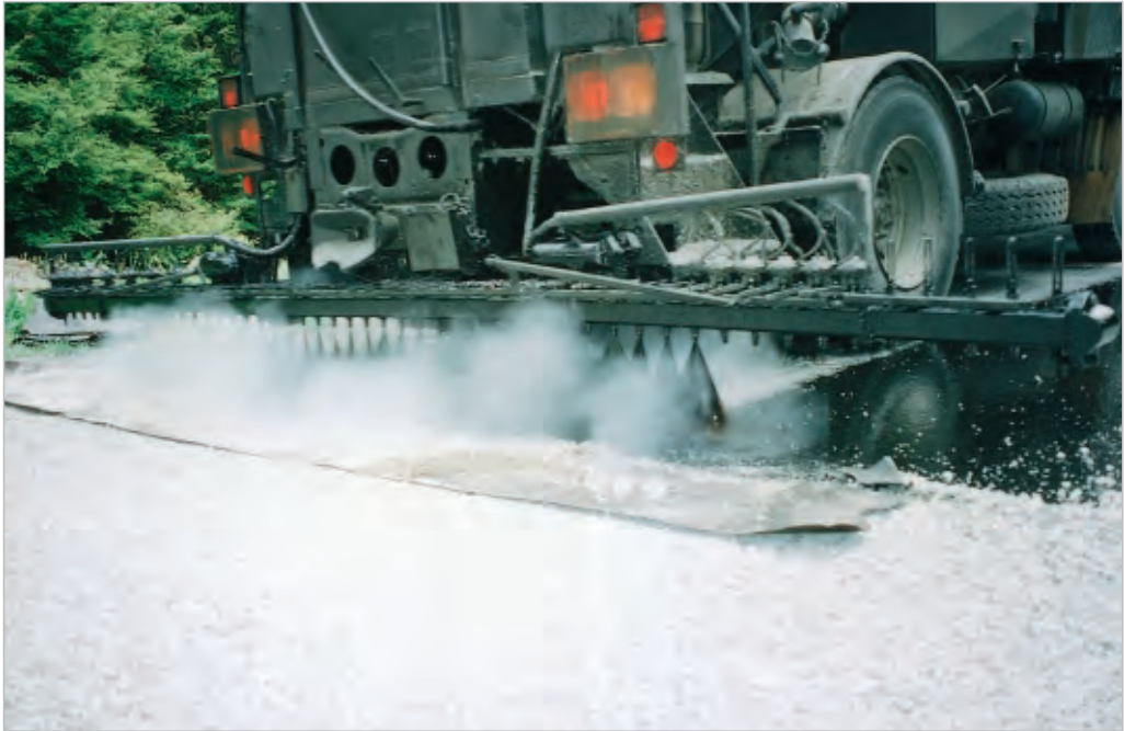
Figure 10-10 Use paper to make an accurate start line when starting a spray run.
