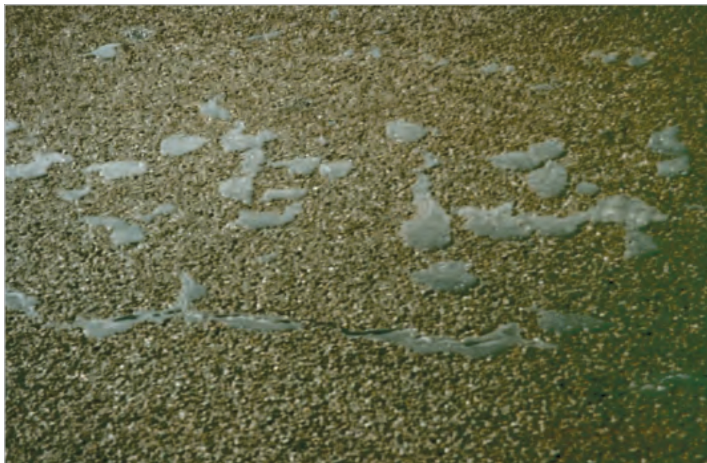
Figure 7-10 Flushing which has reflected through an asphaltic concrete surface.
