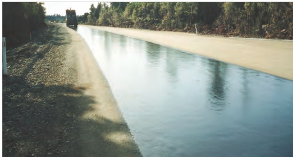
Figure 3-9 A first coat seal under construction on a road on the West Coast of the South Island.
