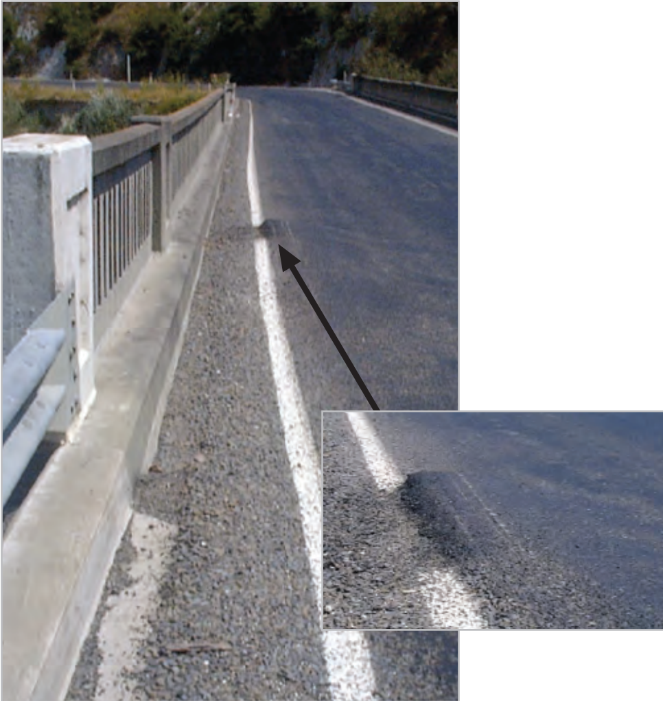
Figure 4-19 Shear failure on a bridge deck.
