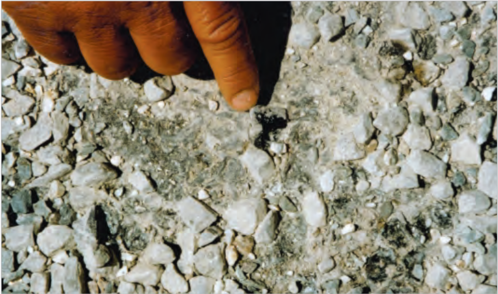
Figure 3-32 Chip loss caused by dirty chip.
