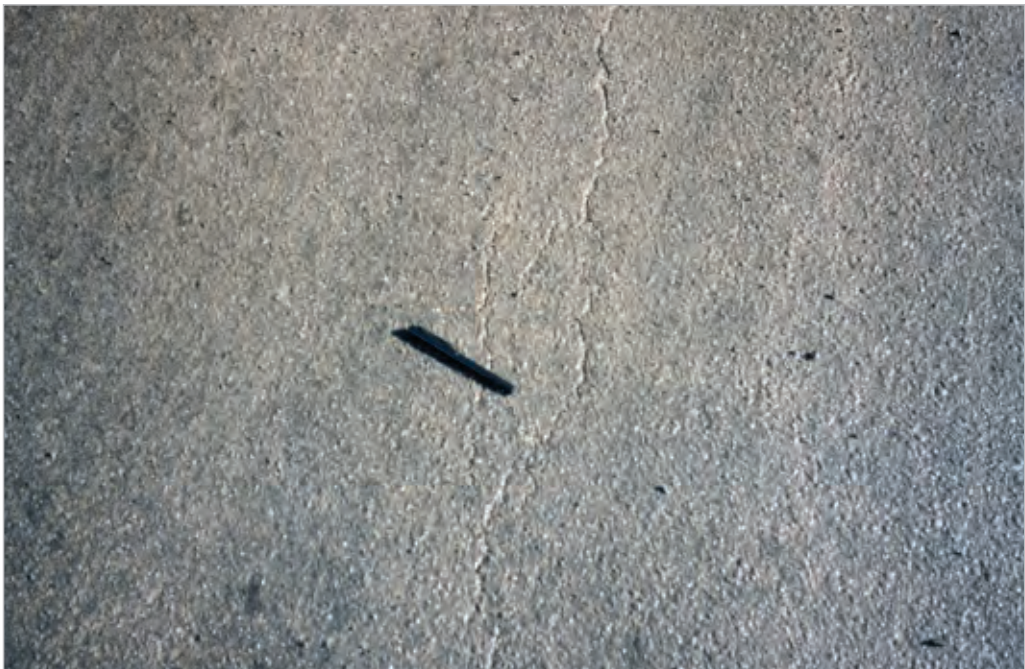
Figure 3-31 Longitudinal and transverse cracks run along or across the road.
