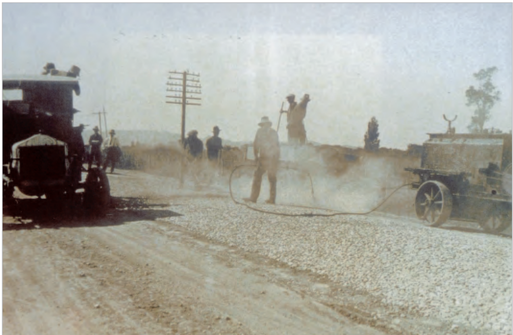
Figure 11-7 In the 1920s, hand spraying was the only way to get the binder onto the road. It required highly developed skills to apply the binder evenly over the surface.
