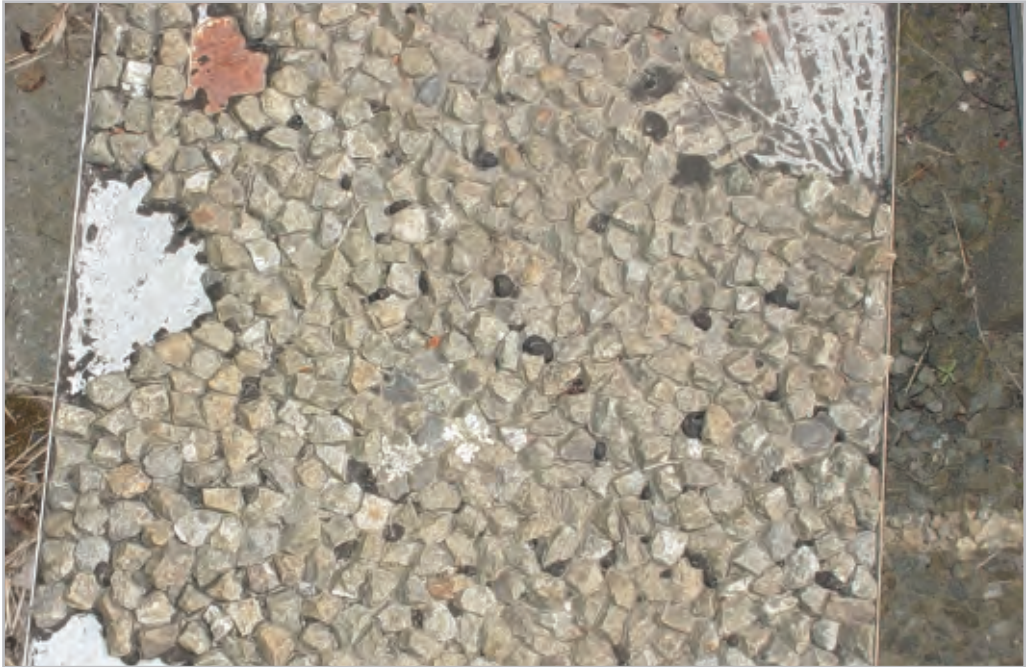
Figure 4-21 Binder rise in a chipseal constructed on a steel plate, for bitumen durability trials at Opus Central Laboratories, Lower Hutt. Samples have been taken from the bare sites.
