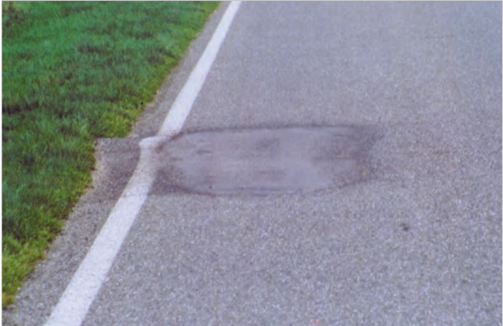
Figure 3-28 Shoving in a pavement.
