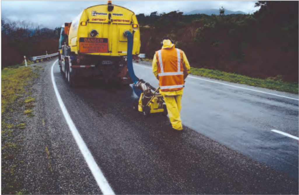
Figure 7-11 A road surface undergoing high pressure water treatment as a repair for flushing.
