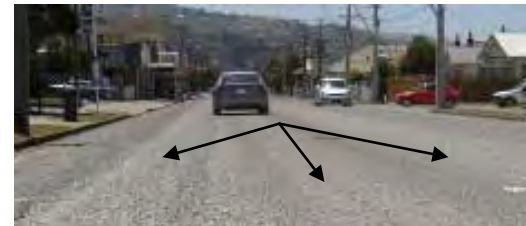
Too much loose chip on seal surface and on road shoulder
