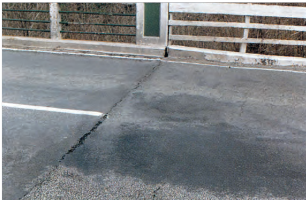
Figure 6-10 Differential settlement of the earthfill at the abutment (from Transit NZ 2001).
