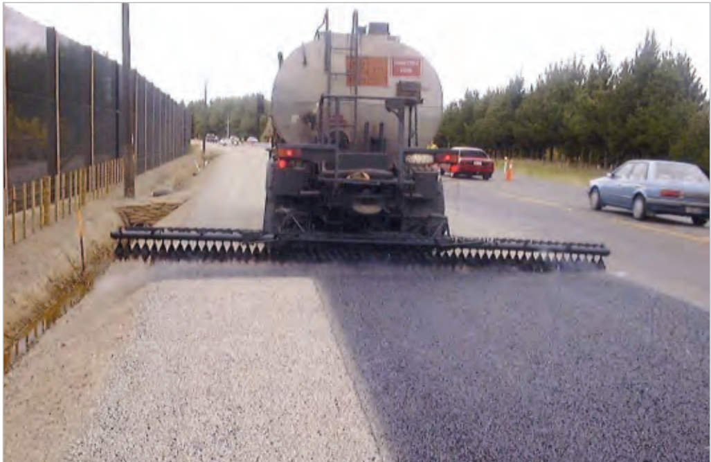
Figure 10-7 Tilting of the spraybar caused by soft suspension. Photo courtesy of DCS Penny Ltd
