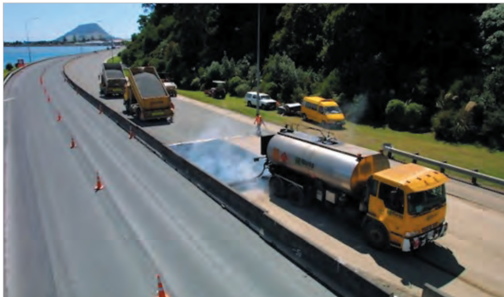
Figure 6-2 A first coat seal is laid on the highway around Tauranga Harbour, Bay of Plenty. The distributor (right) is laying the binder, followed by the chip spreader (reversing over the chips newly laid on the binder). Rolling to compact the chips into the binder will follow. Photo courtesy of Philip Muir, Works Infrastructure
