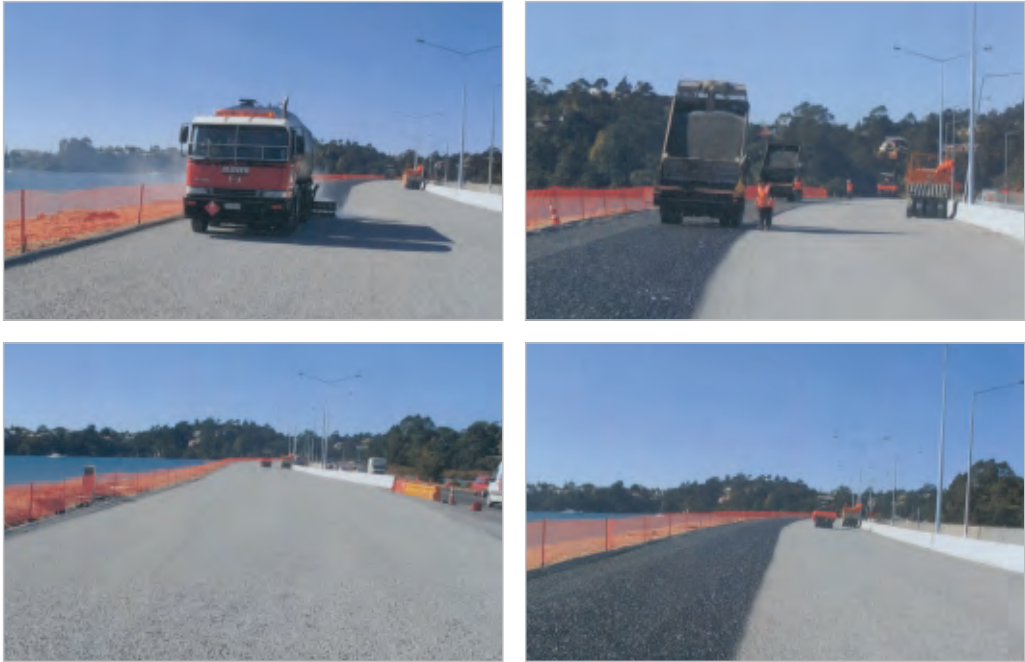
Figure 11-5 Once the planning has been done, seal construction can begin. Clockwise from top left: Spraying the binder. Top right: Spreading the chip. Bottom right: Rolling underway while waiting for the chip-spreading operation to complete the second run. Bottom left: Rolling underway on the almost completed seal. Photos courtesy of David Ashby, Opus
