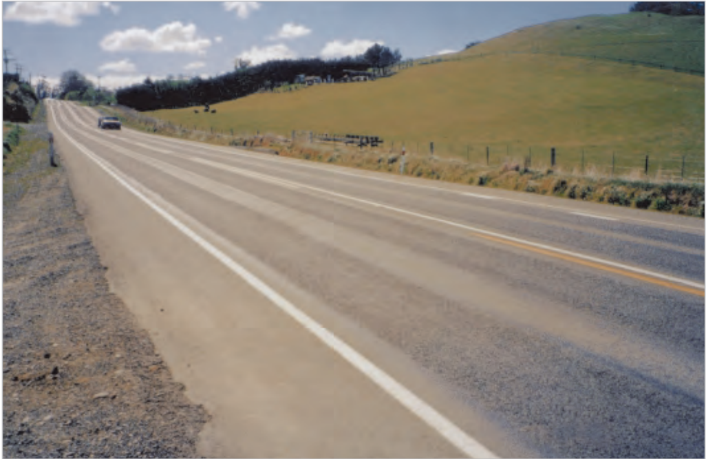
Figure 7-6 These ruts have been filled with slurry, after which the entire surface will be chipsealed. Photo courtesy of Barry Gundersen, Gundersen Consulting Ltd
