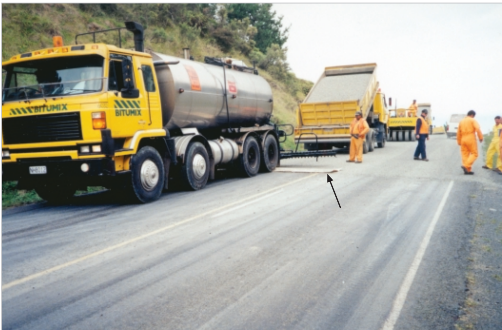
Figure 11-6 A spray run about to start. Note the paper spread in place so that an accurate start line can be achieved. Photo courtesy of Les McKenzie, Opus
