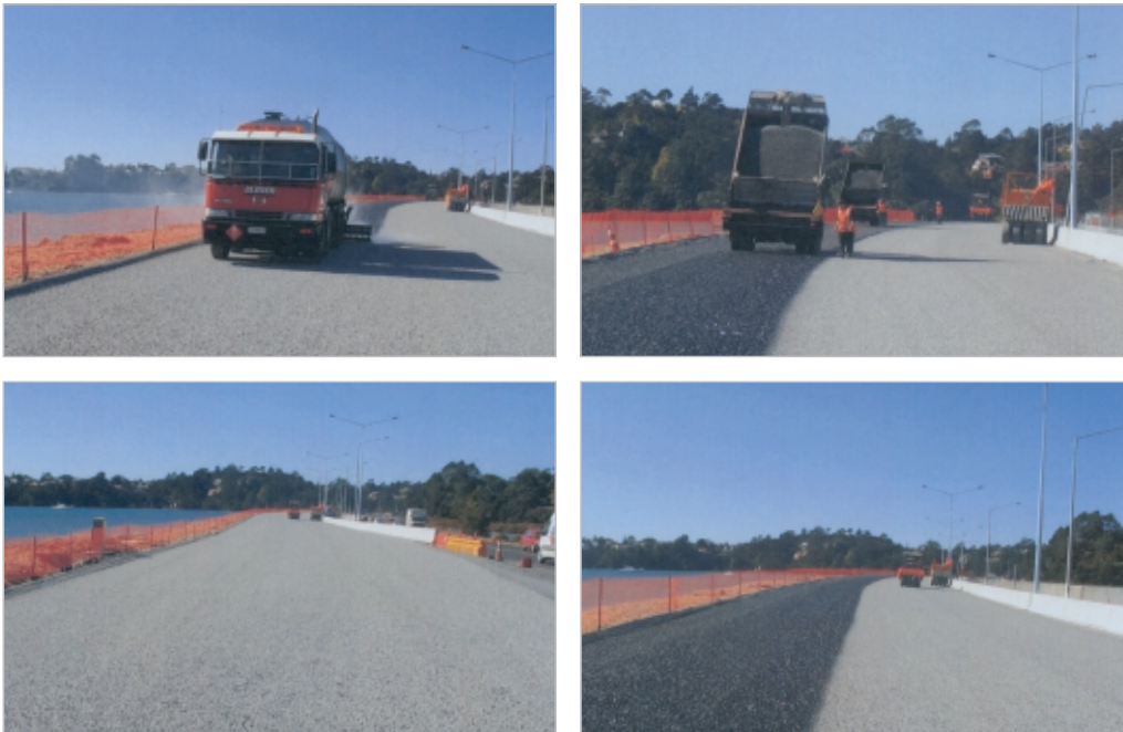
Figure 11-5 Once the planning has been done, seal construction can begin. Clockwise from top left: Spraying the binder. Top right: Spreading the chip. Bottom right: Rolling underway while waiting for the chip-spreading operation to complete the second run. Bottom left: Rolling underway on the almost completed seal.
