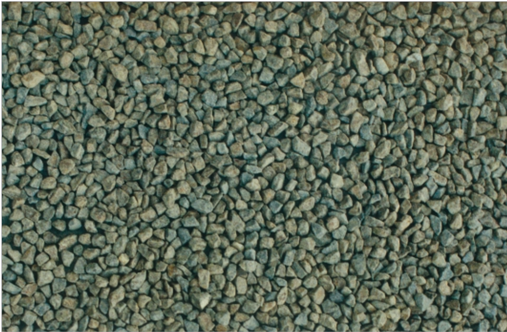
Figure 11-3 Previously advice was to aim for a chip spread-target rate as shown at the top of this page. This is now considered as over-chipping. The image at the bottom of the page shows a very over-chipped seal.
