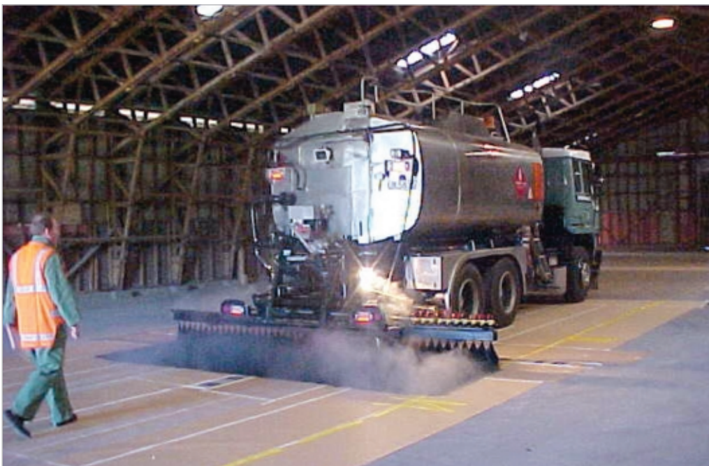
Figure 10-12 Calibration of bitumen distributor. Photo courtesy of Bryan Pidwerbesky, Fulton Hogan Ltd
