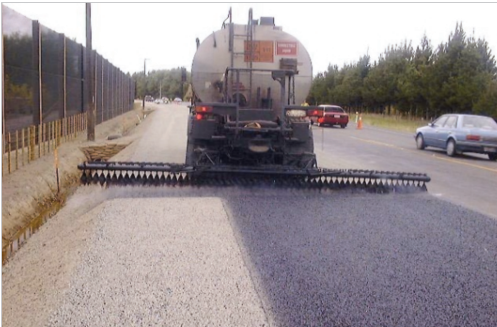
Figure 10-7 Tilting of the spraybar caused by soft suspension. Photo courtesy of DCS Penny Ltd
