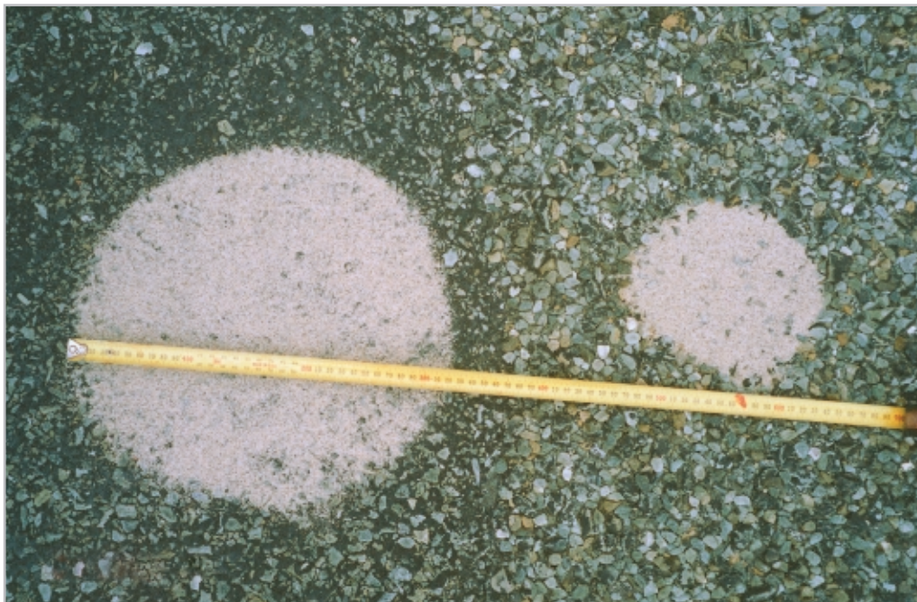
Figure 9-1 Sand circle test is used to determine the texture depth. Comparison of sand circles before (left) and after (right) a Grade 2/4 sandwich seal has been laid.
