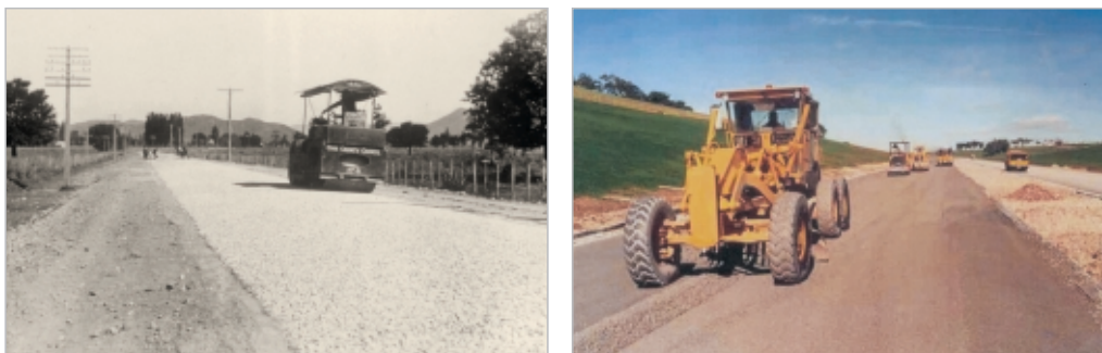
Figure 7-2 Preparation of basecourse for chipsealing has changed a great deal in the last 80 years. Left: A steam roller compacts a new basecourse on State Highway 2 near Manutuke, Cook County, Gisborne, in the 1920s. Photo courtesy of John Matthews, Technix Group Ltd Right: A basecourse to comply with the TNZ B/2:1997 specification is prepared on the Alpurā A2 section of State Highway 1, Auckland in 1999. Photo courtesy of Philip Muir, Works Infrastructure Ltd
