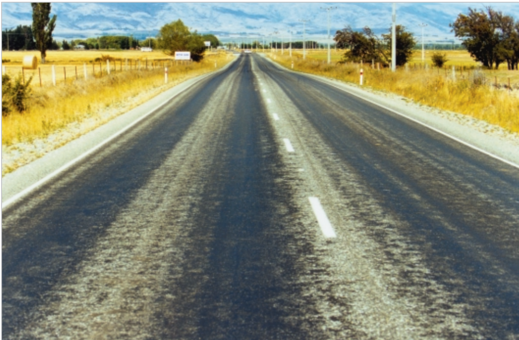
Figure 7-8 A surface in which the wheelpaths have flushed. Note evidence of vapour venting (many small circles of bitumen) on the surface. Photo courtesy of Mark Owen, Transit NZ
