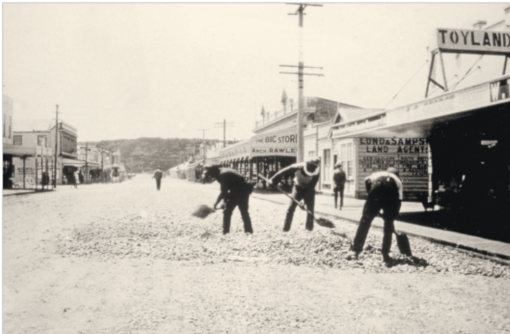
Figure 7-4 Even when chipsealing was less common, failures soon after pavement construction occurred, as they may do today. Here this road works team repairs a non-compliant section of freshly compacted pavement in the main street of a small New Zealand town in the 1920s.
