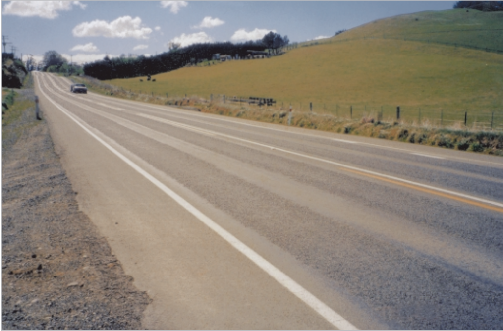
Figure 7-6 These ruts have been filled with slurry, after which the entire surface will be chipsealed. Photo courtesy of Barry Gundersen, Gundersen Consulting Ltd
