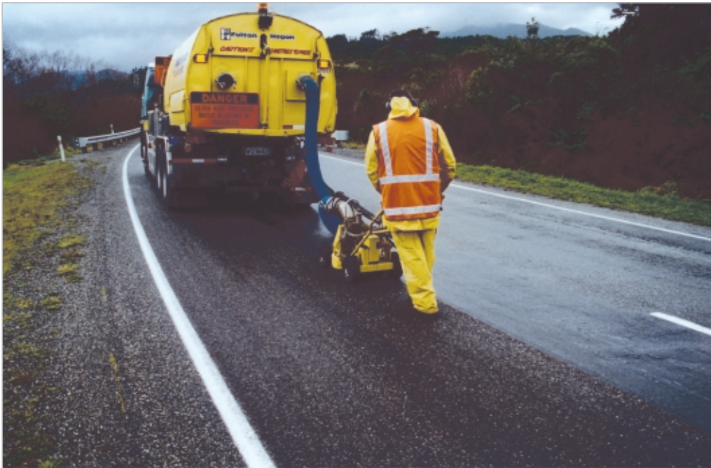
Figure 7-11 A road surface undergoing high pressure water treatment as a repair for flushing.
