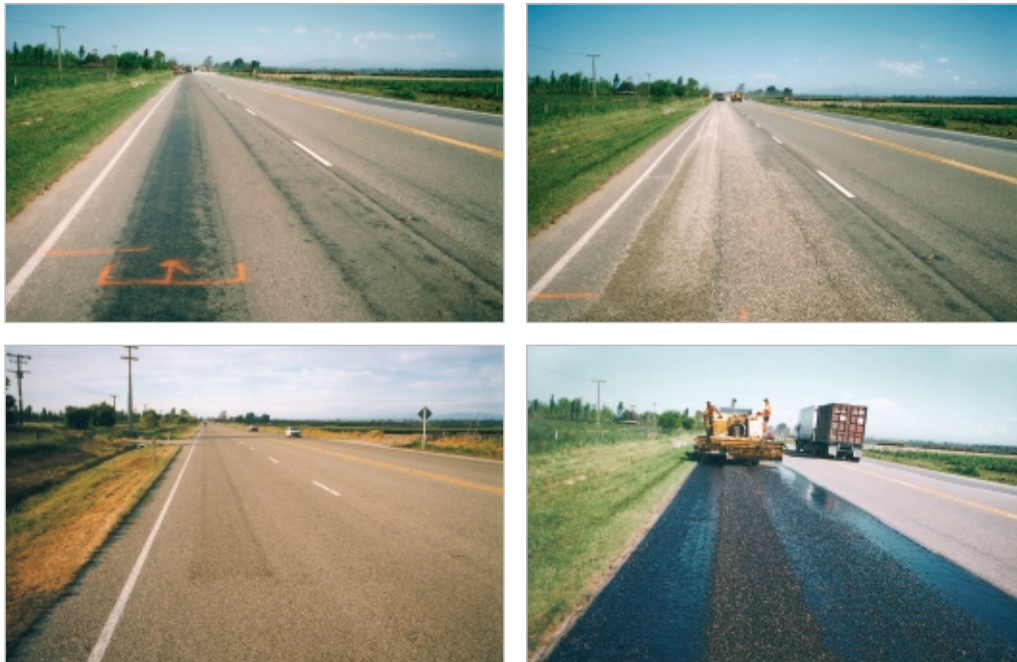
Figure 7-9 Dry chipping a flushed area before chipsealing the entire surface. Clockwise from top left in order of construction: Original surface marked out to show area to be dry chipped. Top right: Dry chip laid in wheelpaths. Bottom right: Binder is laid lane by lane over the dry chip. The next step is to lay the chip over the binder as for a conventional reseal. Bottom left: The completed surface.
