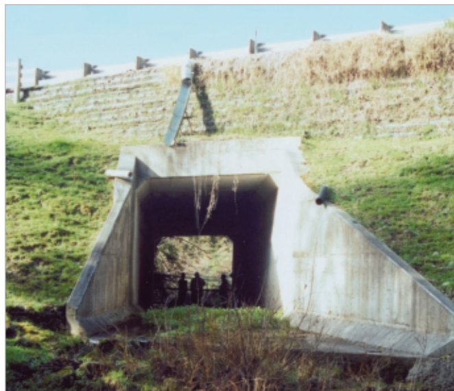
Figure 6-7 An example of a culvert with a high fill. In this case, design of the pavement and surfacing are as for a conventional subgrade (see Section 3.3).
