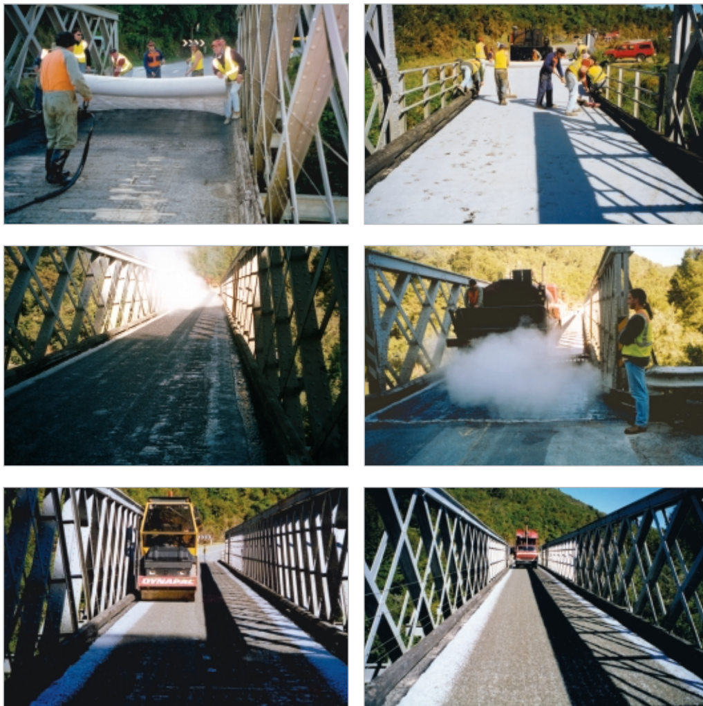
Figure 6-9 A geotextile two coat seal being applied to a single-lane timber bridge (on State Highway 6, West Coast of South Island) to protect joints and metal parts from the effects of water. Clockwise from top left: Laying the geotextile over hand-sprayed tack coat. Top right: Smoothing down the geotextile. Middle right: Spraying the geotextile with the binder. Bottom right: Spreading the chip over the geotextile. Bottom left: Rolling the chip onto the geotextile. Middle left: Spraying the second application of binder over the geotextile and first chip layer. The next step is to apply a second layer of chip.
