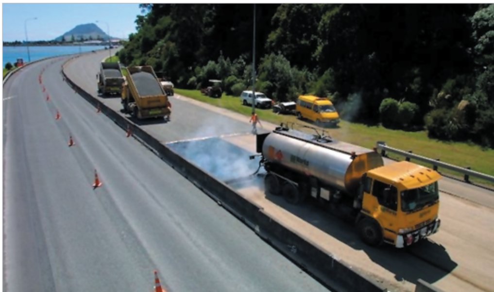
Figure 6-2 A first coat seal is laid on the highway around Tauranga Harbour, Bay of Plenty. The distributor (right) is laying the binder, followed by the chip spreader (reversing over the chips newly laid on the binder). Rolling to compact the chips into the binder will follow. Photo courtesy of Philip Muir, Works Infrastructure
