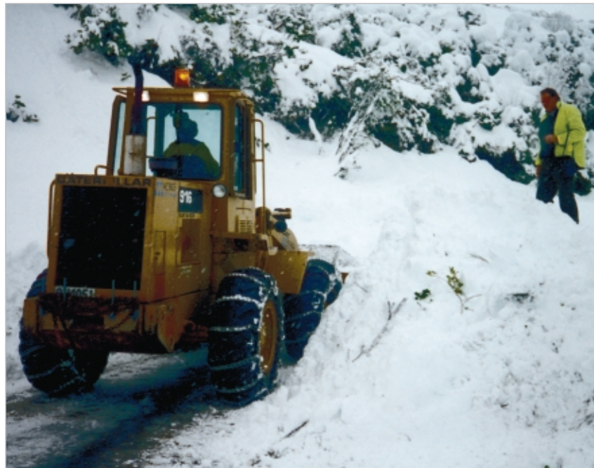
Figure 6-16 Snow clearing with graders and loaders (with wheel chains) can cause damage to the chipseal. Photo courtesy of Les McKenzie, Opus
