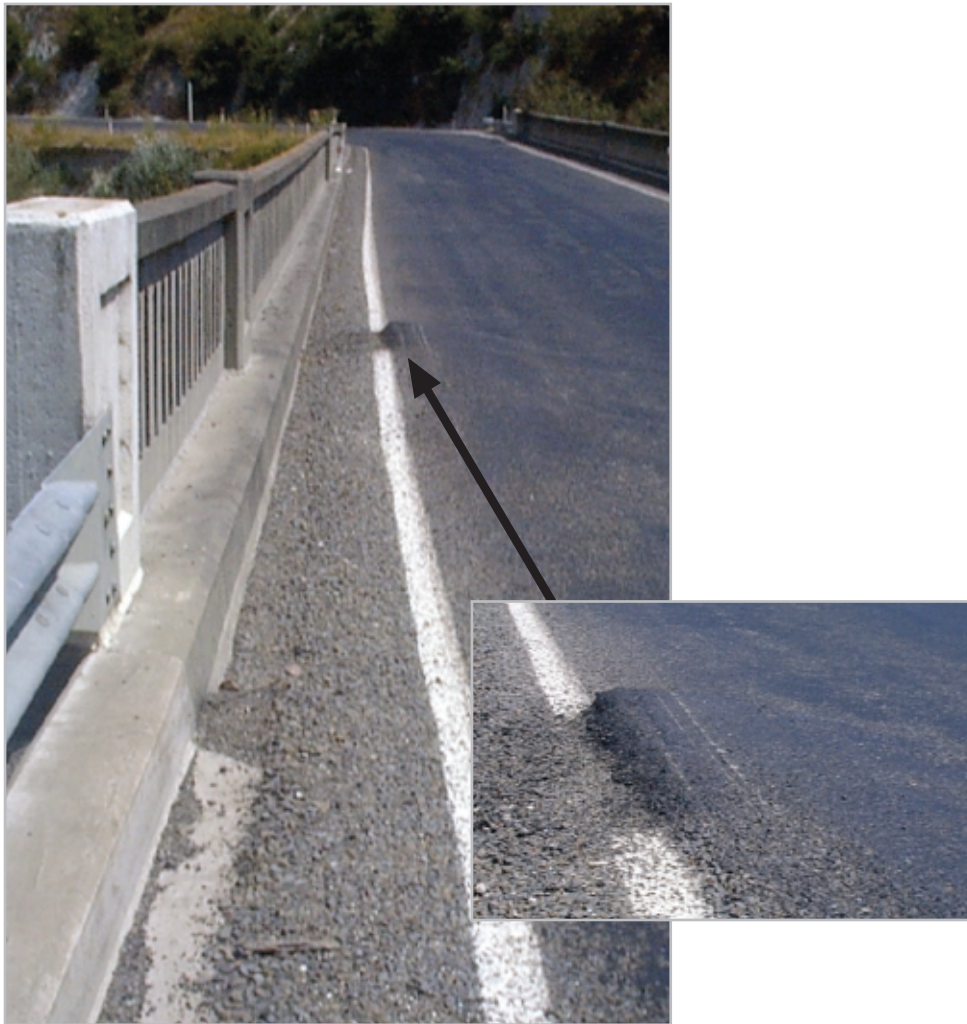
Figure 4-19 Shear failure on a bridge deck.
