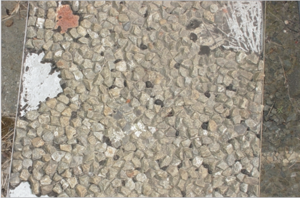
Figure 4-21 Binder rise in a chipseal constructed on a steel plate, for bitumen durability trials at Opus Central Laboratories, Lower Hutt. Samples have been taken from the bare sites.
