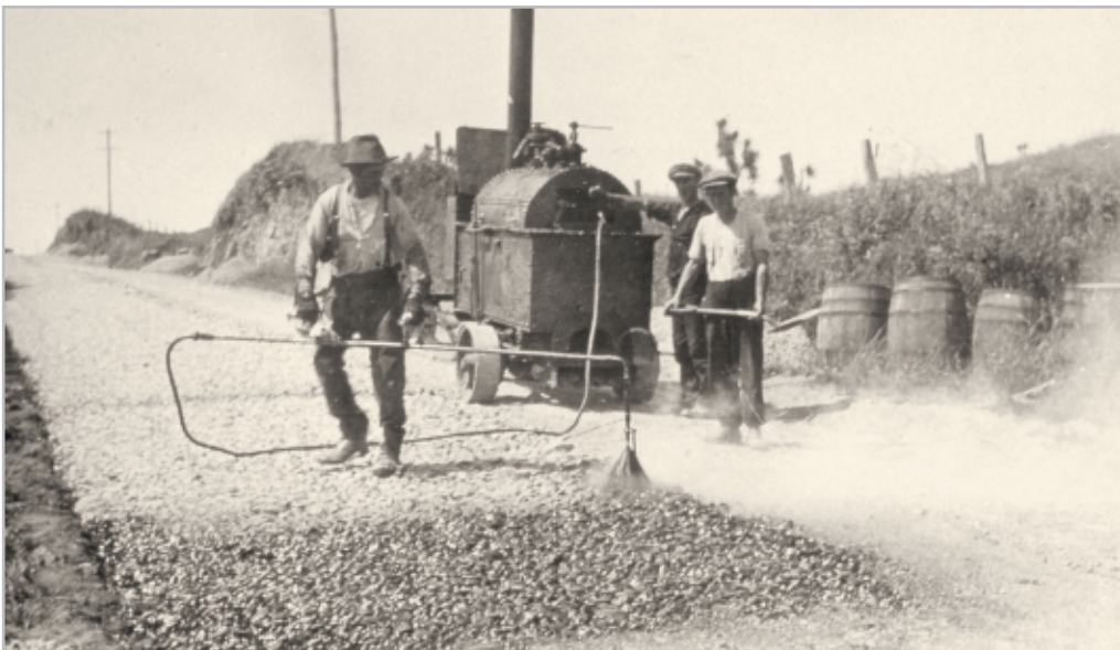
Figure 1-5 Most early chipsealing was carried out to keep down dust in the summer and mud in winter. In the 1920s this spray operator in Opunake County was using a hand sprayer with a swinging boom that kept the hose clear of the hot bitumen tank. Photo courtesy of John Matthews, Technix Group Ltd
