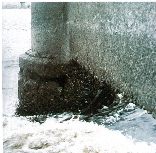
Figure 9.1: Abrasion of concrete pile cap.
