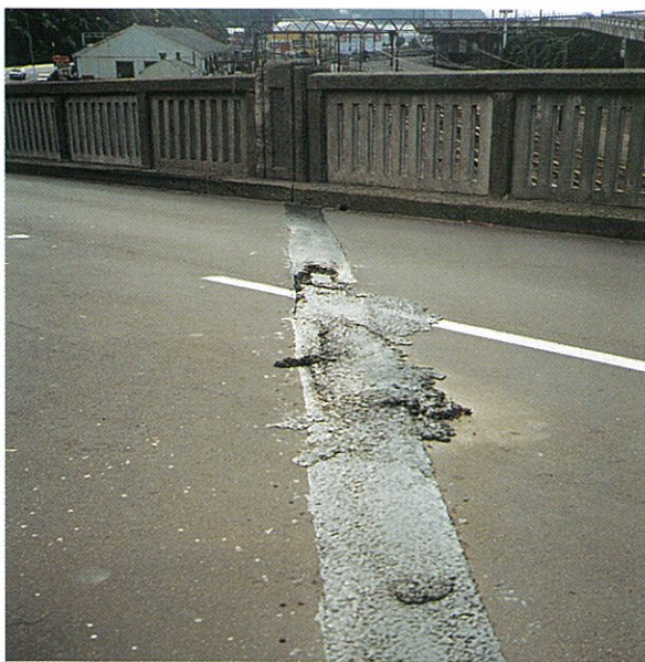
Figure 8.5: Asphaltic plug joint skewed to the traffic flow showing flow of joint material out of recess due to traction forces.
