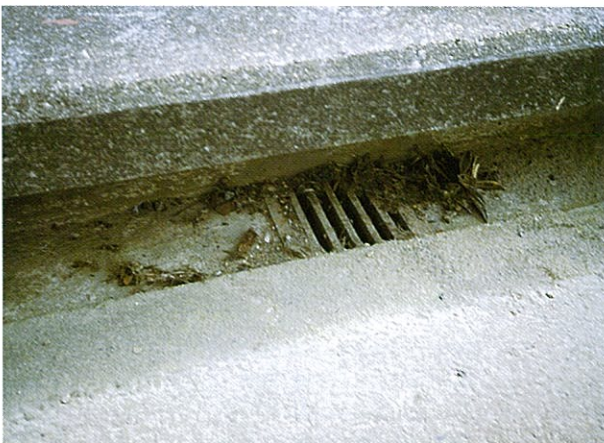
Figure 7.1: Small grates require frequent maintenance.
