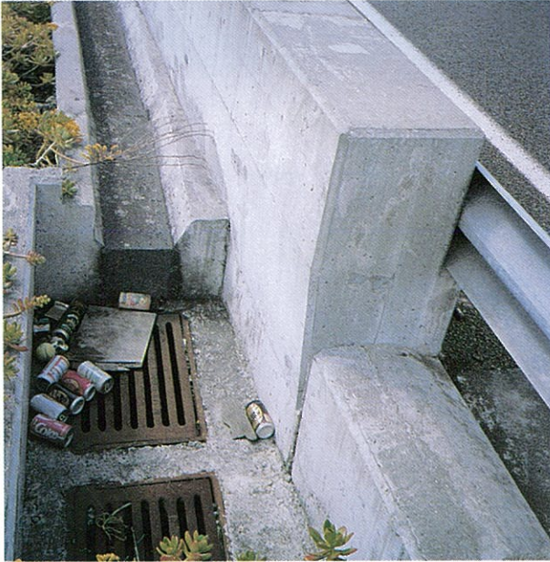
Figure 7.2: Typical debris collecting on grate.
