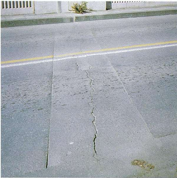
Figure 7.5: Leaking deck joint.
