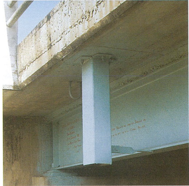
Figure 7.4: Drainage outlet below adjacent steel beam soffit.
