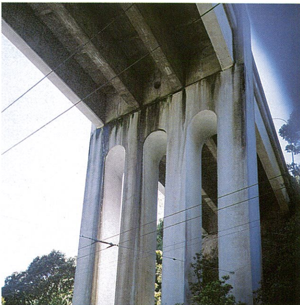
Figure 7.6: Staining of pier caused by leaking deck joint.
