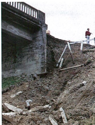
Figure 6.3: Failure caused by seepage and poor drainage.
