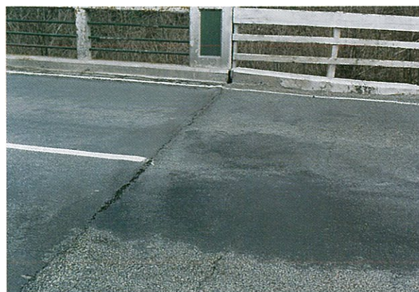
Figure 6.1: Settlement of approach caused by lack of fill containment.
