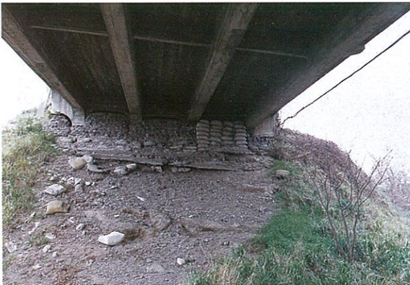
Figure 6.2: Ineffective fill containment.
