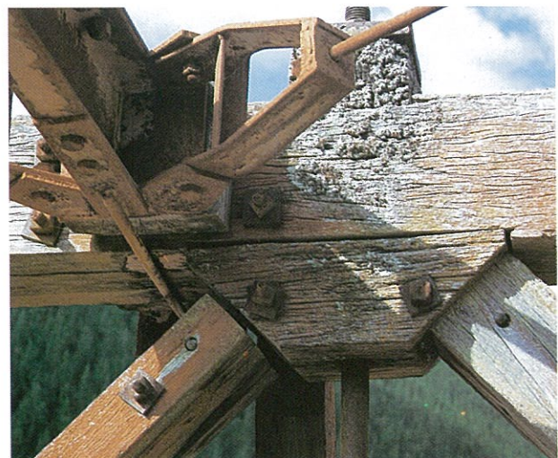
Figure 5.11: Joint defects: movement from compression, looseness of tension member, open holes from investigation drilling, corrosion of steel fixings, moss growth and decay.
