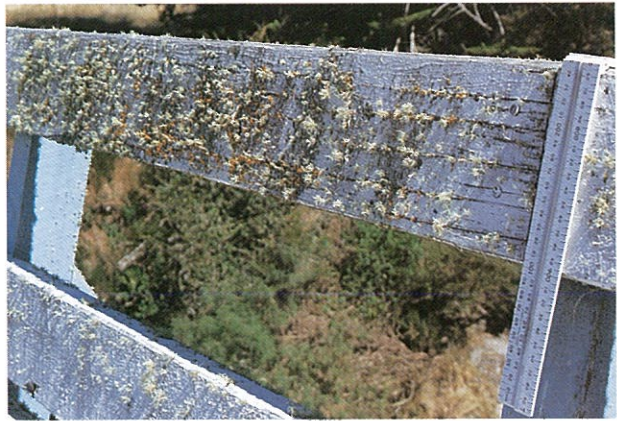
Figure 5.10: Splits in painted macrocarpa rail and moss growth after 10 years.
