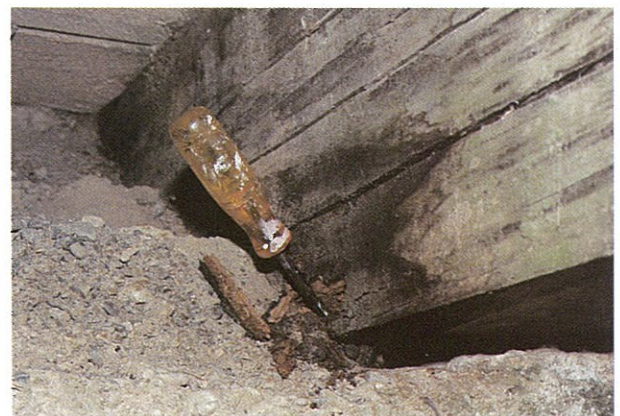
Figure 5.8: Accumulation of gravel, splits and advancement of decay at bearing area of timber beam.
