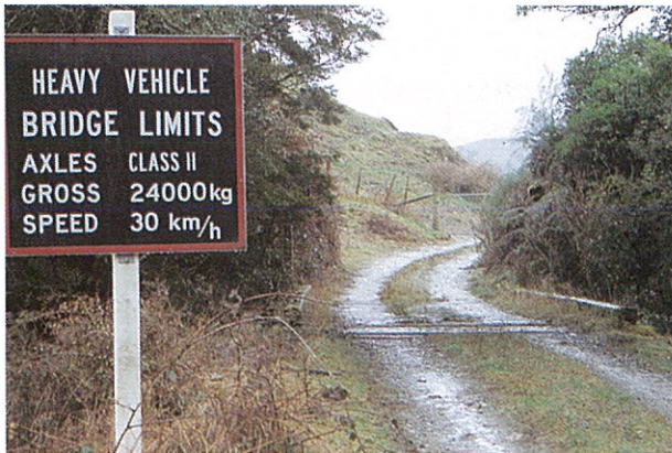
Figure 5.17: Old bridge with load restriction.
