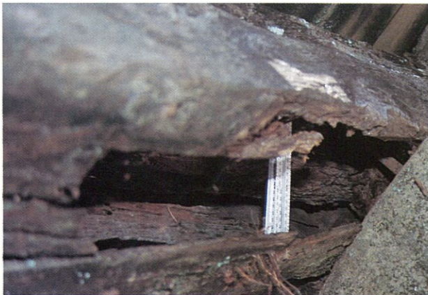
Figure 5.6: Decay is the most serious timber defect.
