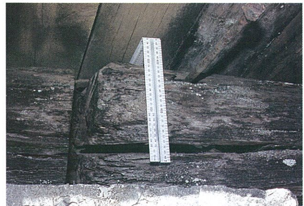
Figure 5.13: Large split at bearing area of beam greatly reducing load capacity in shear.
