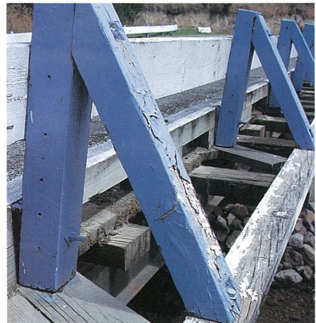
Figure 5.14: Maintaining a sound painted coating is a problem on old timber rails.
