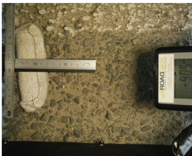
Figure 6. New ATP ribs, with good rib height, in need of cleaning (along with the road surface in this case)
