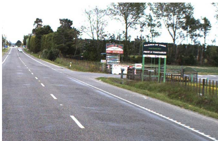
Figure 5. ATP roadmarkings should be omitted from major accessways and intersections but continuous across minor entrances unless noise is a problem for residents
