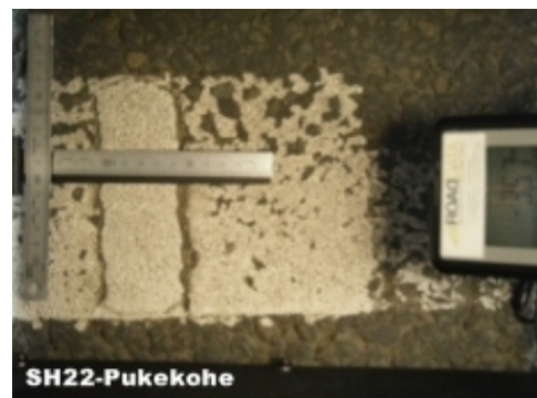
Figure 9. Old ATP that is due for reinstatement
