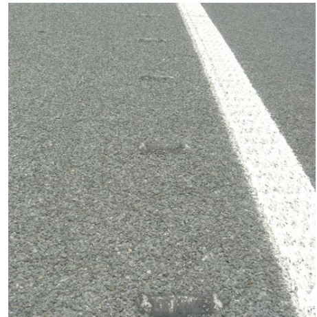
Figure 8. A reseal using a fine grade chip over relatively new ATP ribs. Note the new line has been incorrectly placed and should be immediately adjacent to the ATP ribs
