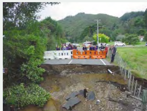
Above: Local interest in watching the Bailey bridge being installed over a washout.
