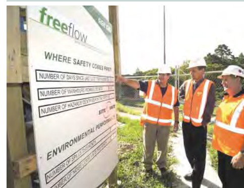
Freeflow health and safety manager Jonathan Pauro, Transit chief executive Rick van Barneveld and environmental control manager Rowan Smiley assess the safety billboard at the Grafton Gully Project.
