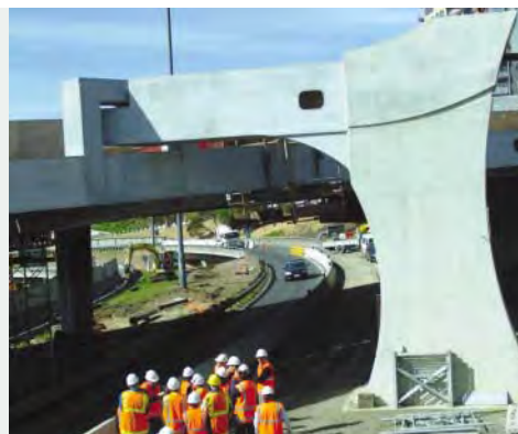
Specially designed outrigger piers support the newly widened motorway. The piers enable traffic below to flow uninterrupted and height clearances to be maintained.
