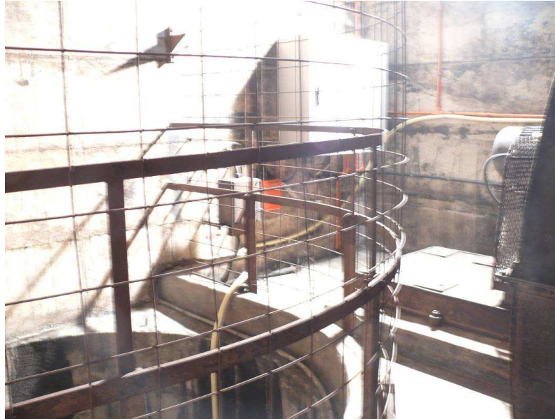
Figure 38: The interior of the Mt Victoria Tunnel western exhaust stack building showing the top of the exhaust vent (below left) and the sampling duct passing from the duct along the wall to the trailer at the exterior of the building.
