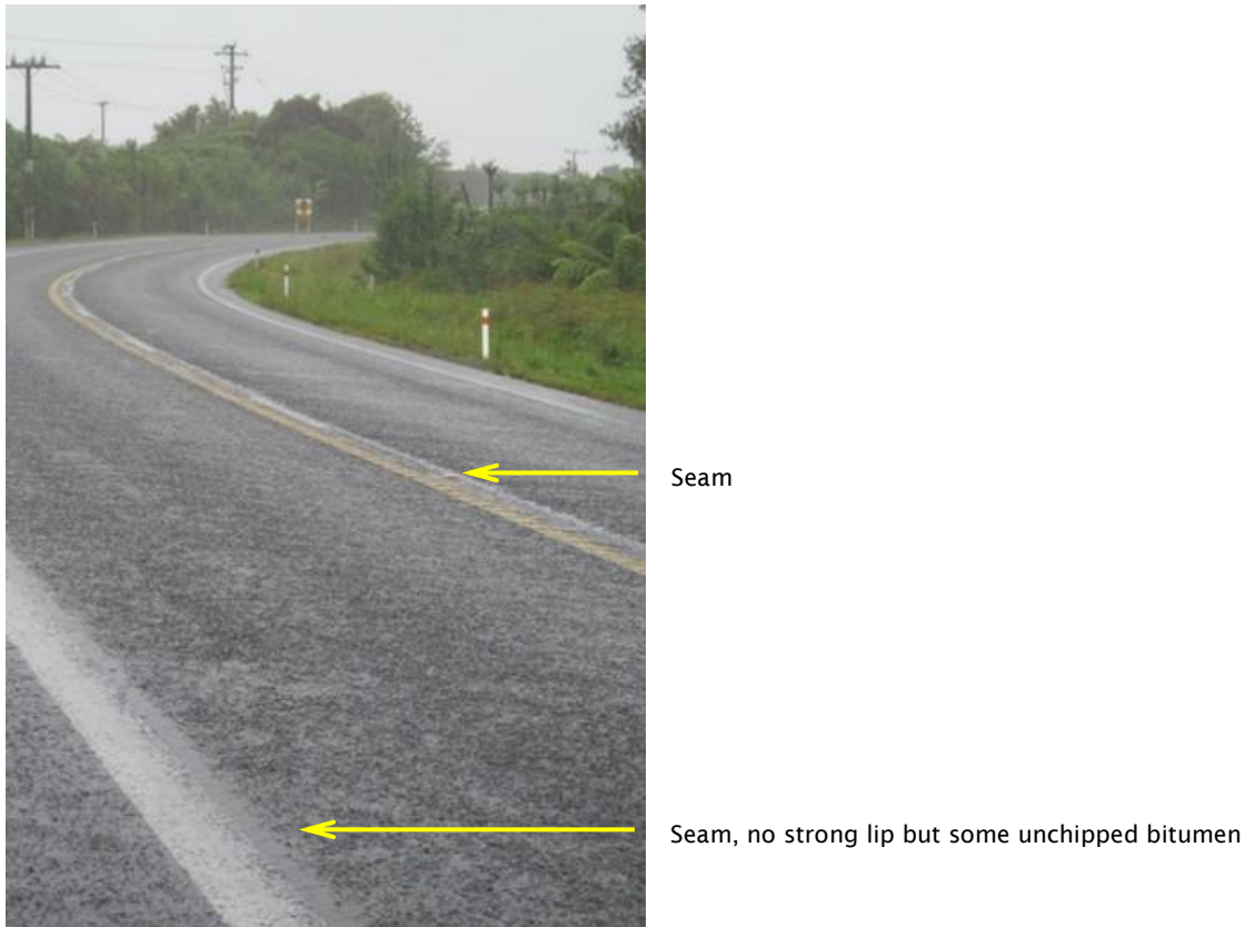
Figure 2.3 Example of an in-lane reseal seen in heavy rain and with lighting conditions highlighting water ponding/accumulation 4
