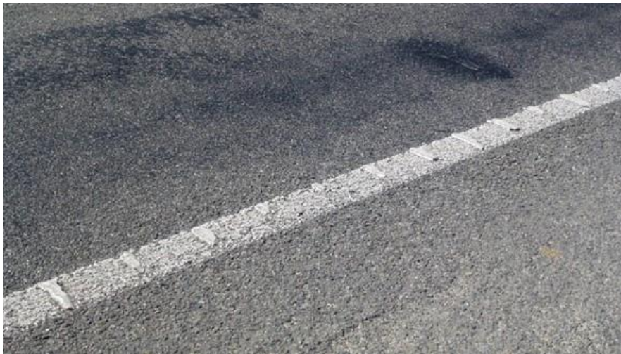
Figure 4.15 ATP roadmarkings damaged by snowploughing (example 6)
