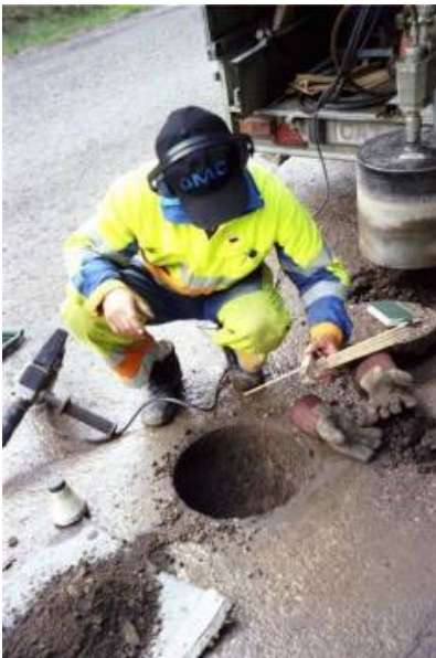
Figure A.13 Sampling of unbound basecourse sample, which is then stored normally in plastic bags
