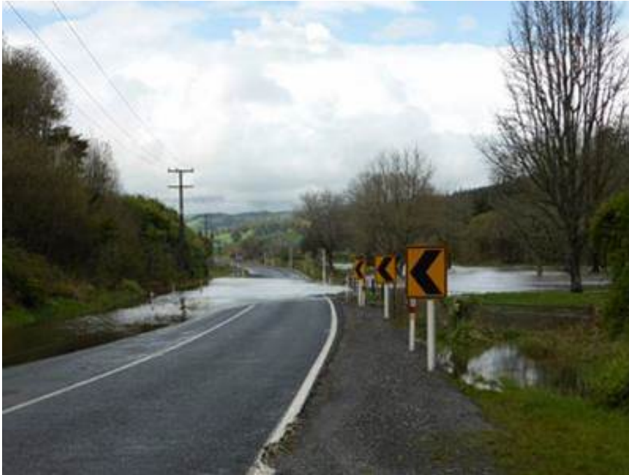
Figure A.1 Heavy rainfall and an inadequate drainage system can cause flooding and erosion around and under the road pavement. Water infiltrating the pavement structures also reduces the stiffness and bearing capacity of the road and exposes the pavement to permanent deformation
