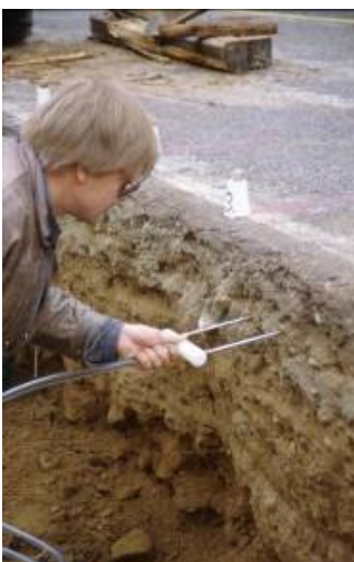
Figure A.17 Installation of a typical TDR probe in road structure (Hänninen 1997)
