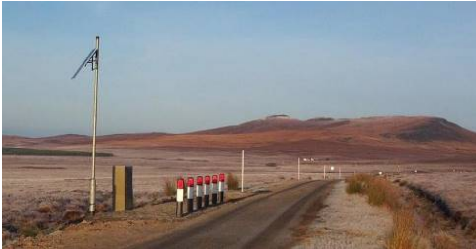
Figure A.15 Percostation installed in road B871 in Scotland
