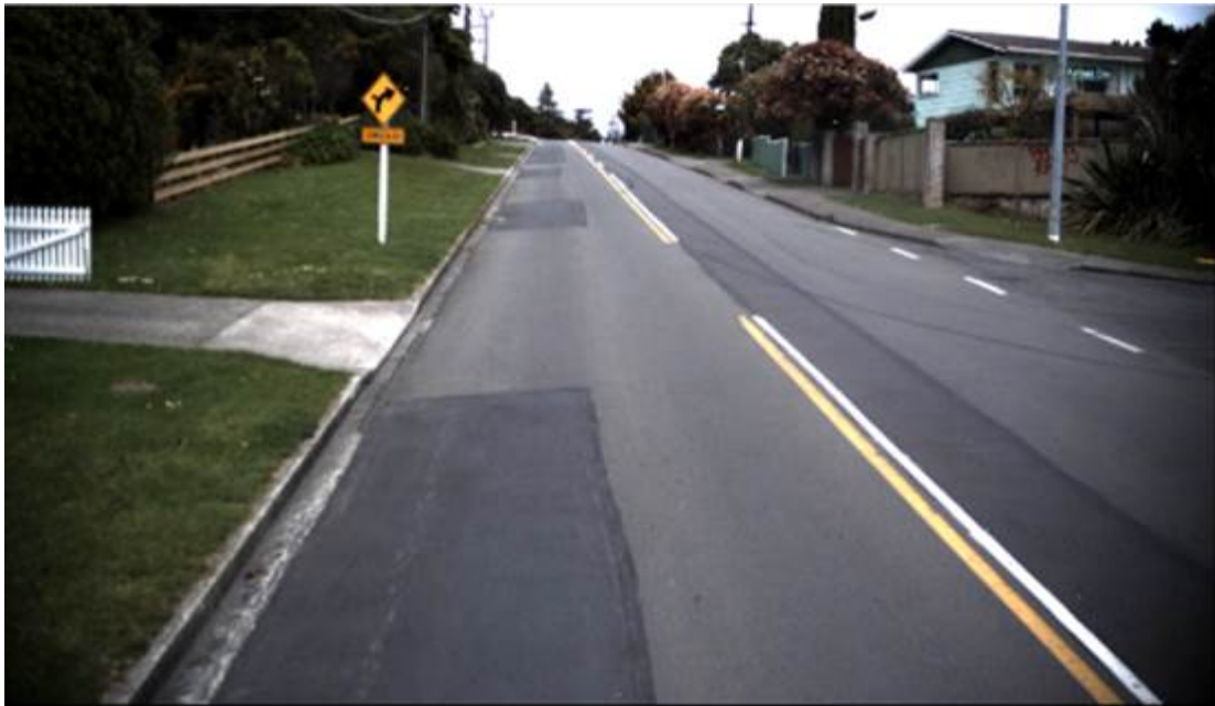
Figure B.5 Moisture survey results on Ruapehu Street spot # 3 (RP approx 688m) - black shade indicates highest level of saturation or MDI
