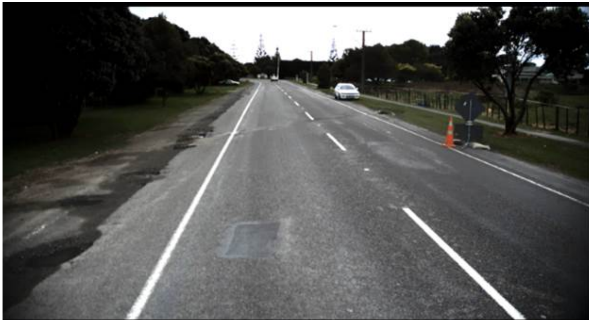
Figure B2.3 Moisture survey results on Te Moana Road spot # 3 (RP approx 3,220m) – black shade indicates highest level of saturation or MDI
