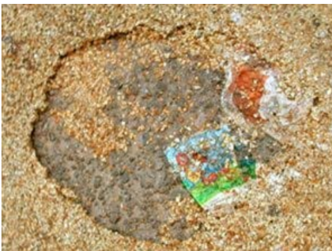
Figure 2.1 Example of delamination in coloured surfacing
