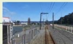
Dowse interchange bypass - south connection • 3.5m-wide cycle path • 1.8m-high security fence and lighting • 1.5m-wide southbound cycle bypass
