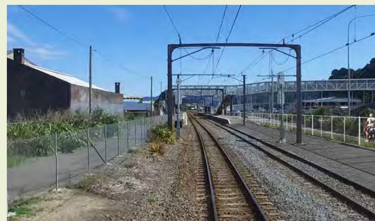
North of Petone railway station ▪ 3.5m-wide cycle path ▪ 1.8m-high security fence and lighting
