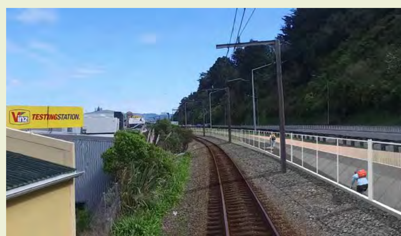
South of Parliament Street rail underpass ▪ 3.5m-wide cycle path ▪ 1.8m-high security fence and lighting ▪ 1.1m-high balustrade to highway ▪ lighting and security cameras integrated with underpass structure
