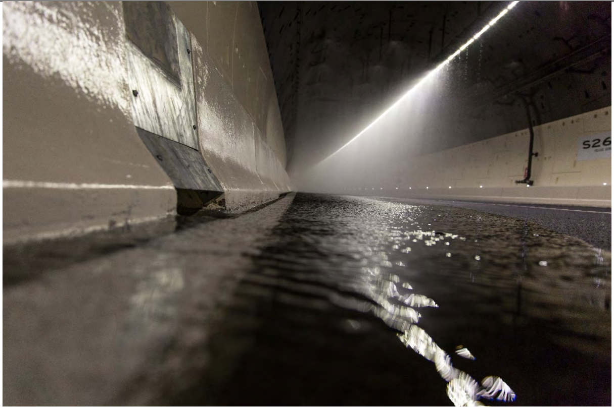
Typical Deluge run off into drain
