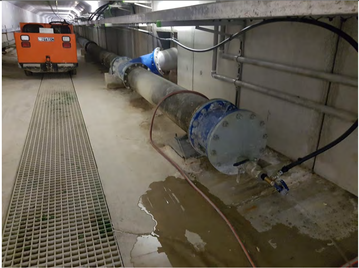
Pipe Work and Sample point at North Bound Culvert XP14
