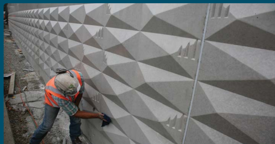
The Westhaven Drive retaining wall typifies the high quality urban design sought by the project.
