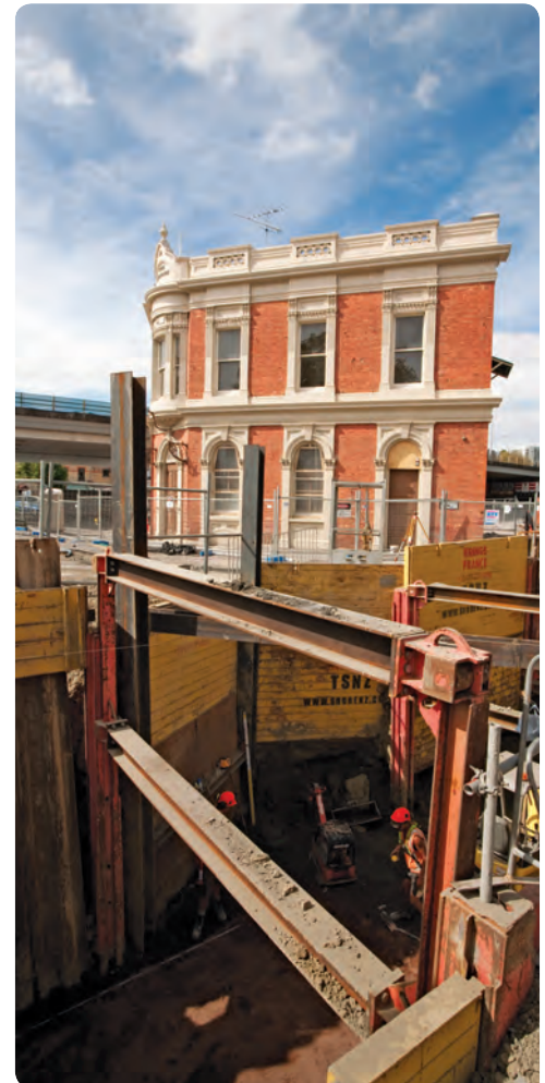
Major services including the Freemans Bay Stormwater Culvert have been moved away from the Rob Roy.
