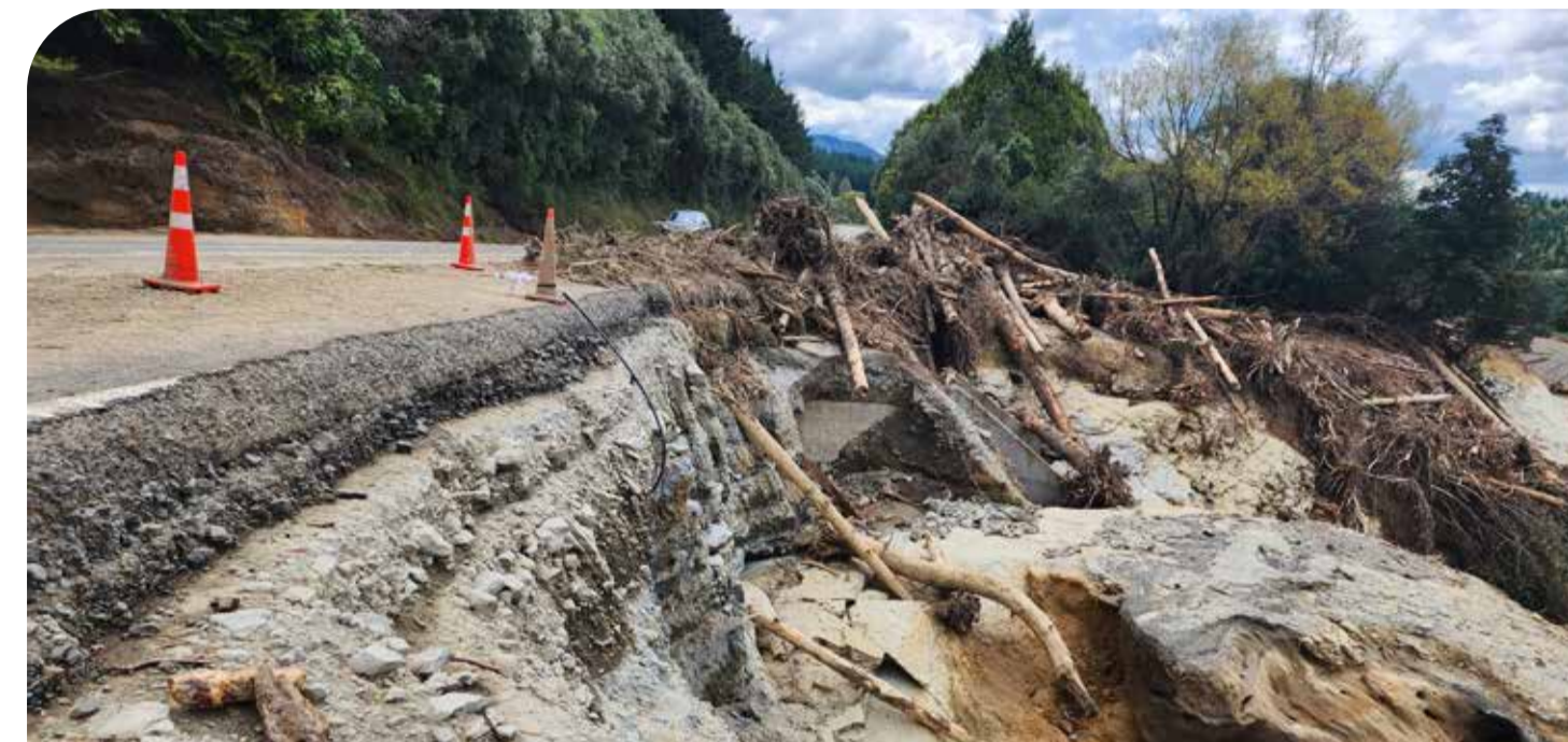
Large underslip at Captain's Culvert
