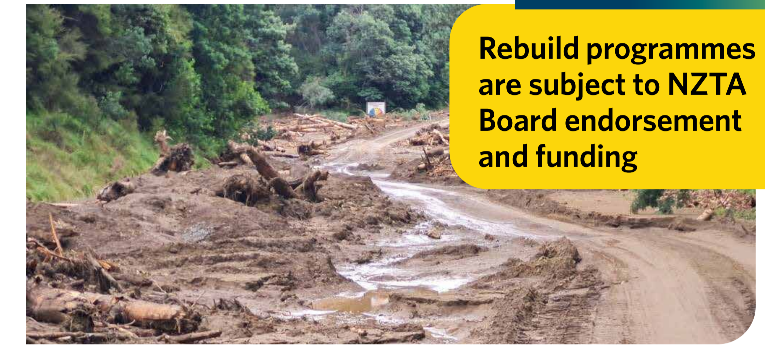
Cyclone damage at SH5 Eland
