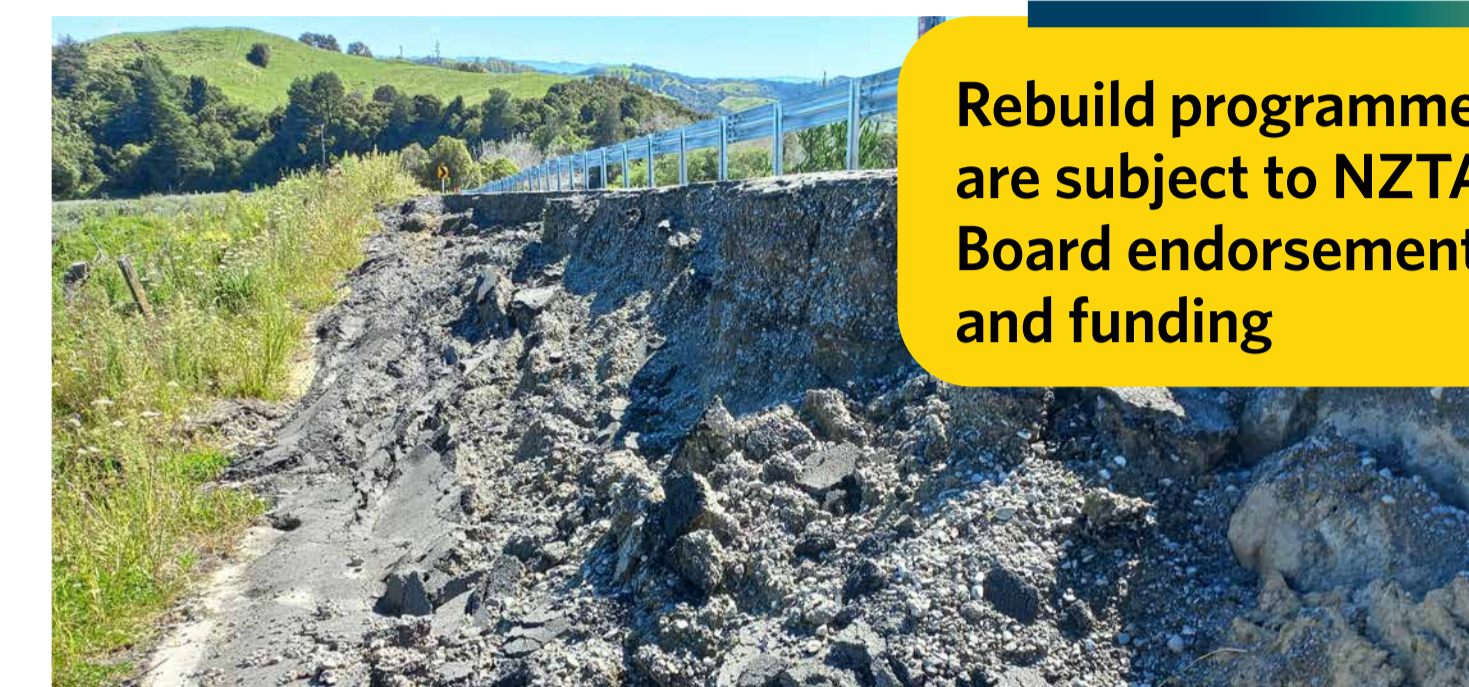
Damage at SH2 Mohaka Hill
