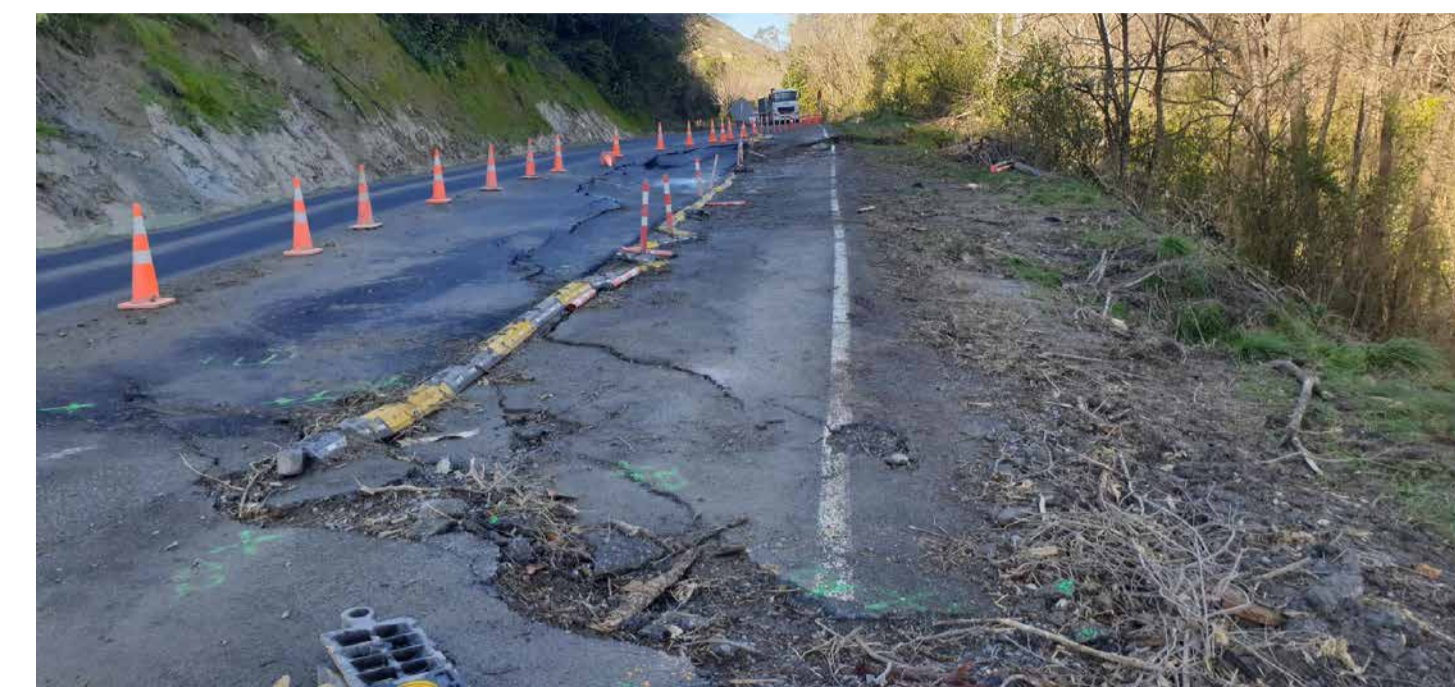
Damage at White Pine Bush
