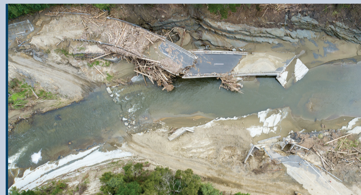
February | The old bridge collapsed during Cyclone Gabrielle
