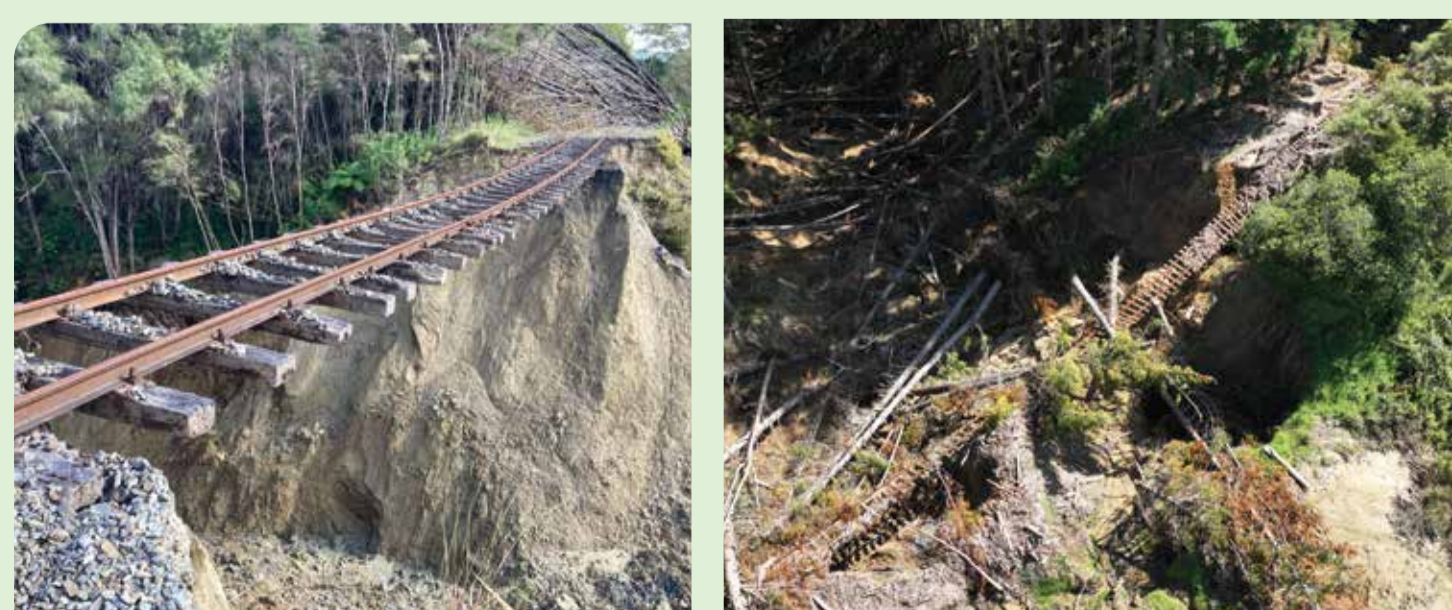
Culvert / embankment failure at PNGL
