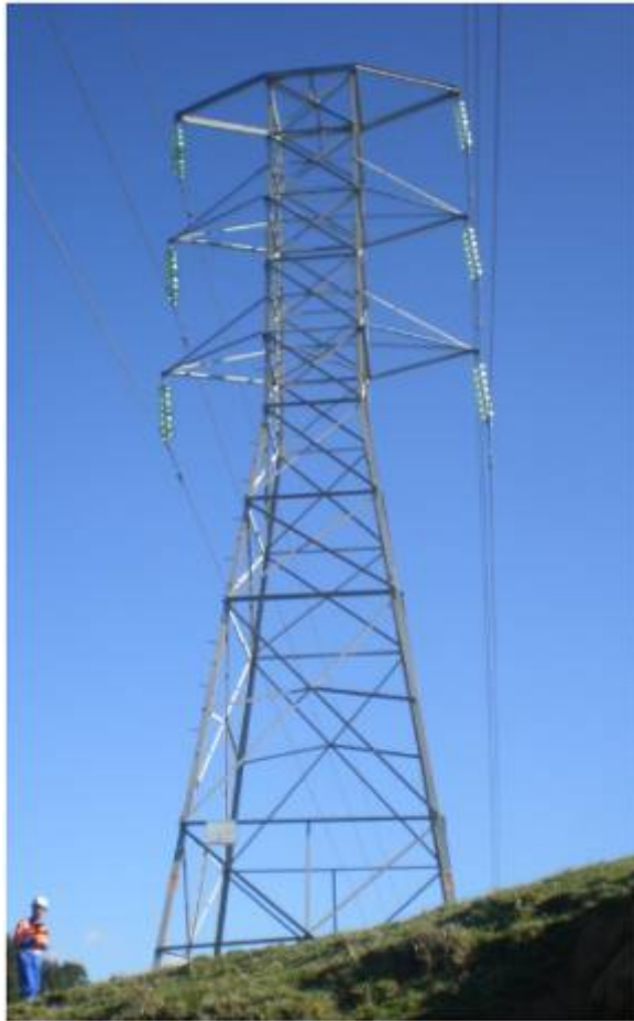
Figure 3.3: Example of a Suspension Tower (PKK-TKR A transmission line).
