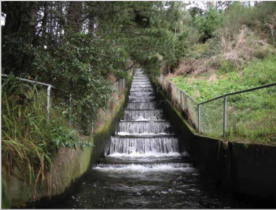
Photo 9-25 Lower Canons Creek concrete steps prior to a perched culvert release into the Kenepuru Stream.
