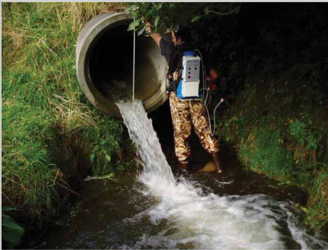
Photo 9-26 The perched culvert releasing Canon's Creek stream to the Kenepuru Stream. (Fish passage barrier).
