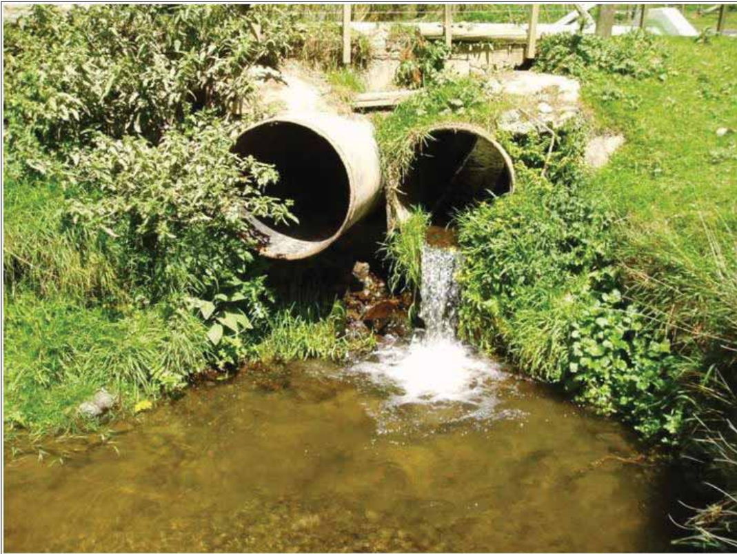
Photo 9-18 One of the three perched culvert arrangements currently in the upper Duck main stem
