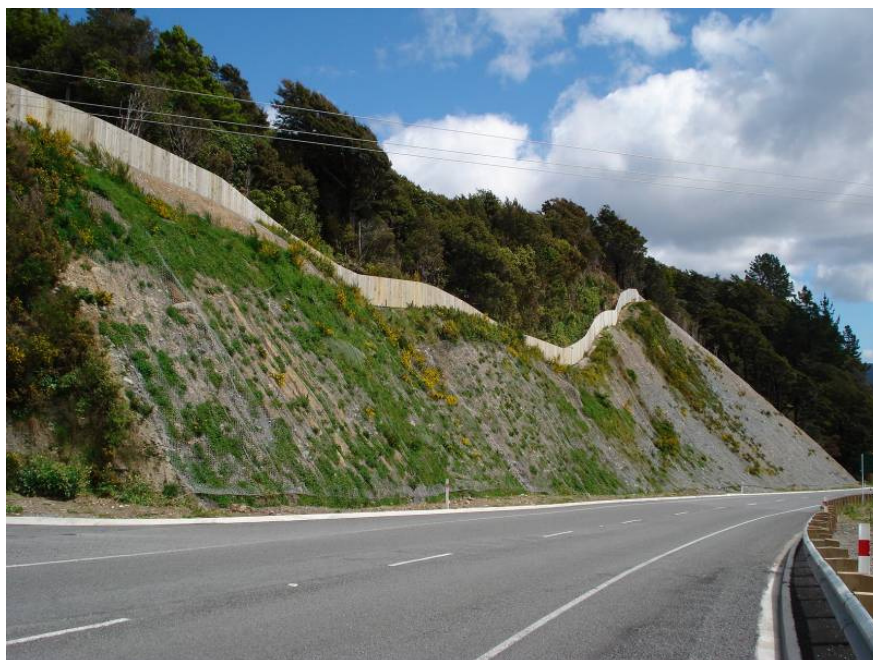
Illustration 3.21 - Rock Fall Protection Netting at SH 2 Kaitoke to Te Marua
