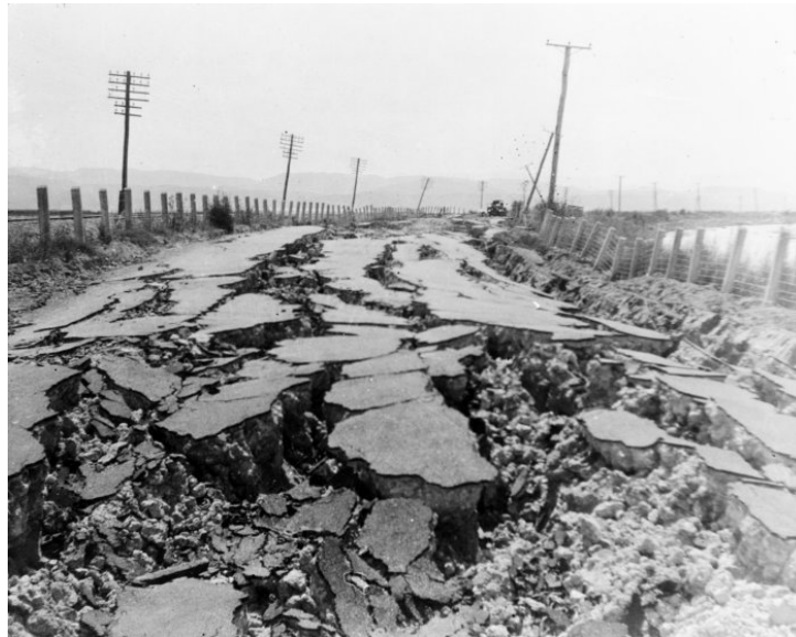
Illustration 3.29 - Failure of Road Embankments due to Liquefaction in 1931 Hawkes Bay Earthquake
