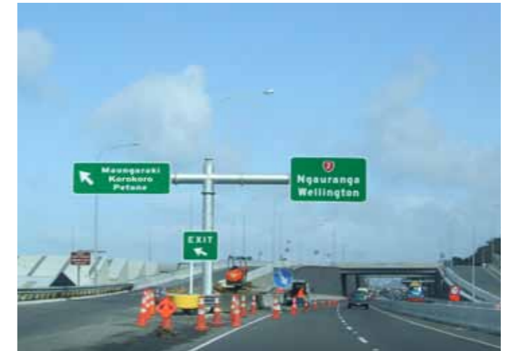
Photo 4.29: Single support signage at off-ramp
