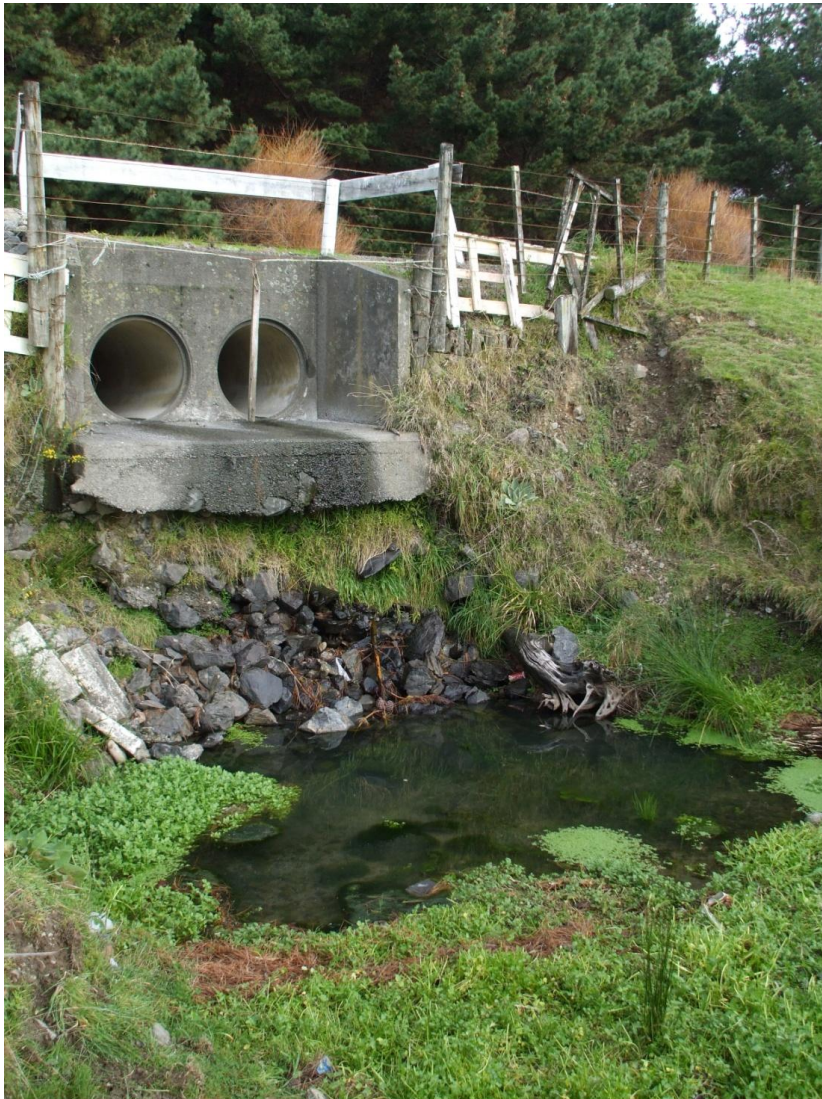
Twin barrel perched culvert of the Wainui arm as it emerges from under State Highway 1.
