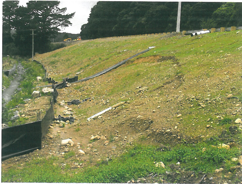
Photograph 4 – Kaitoke realignment embankments after February 2004 storm
