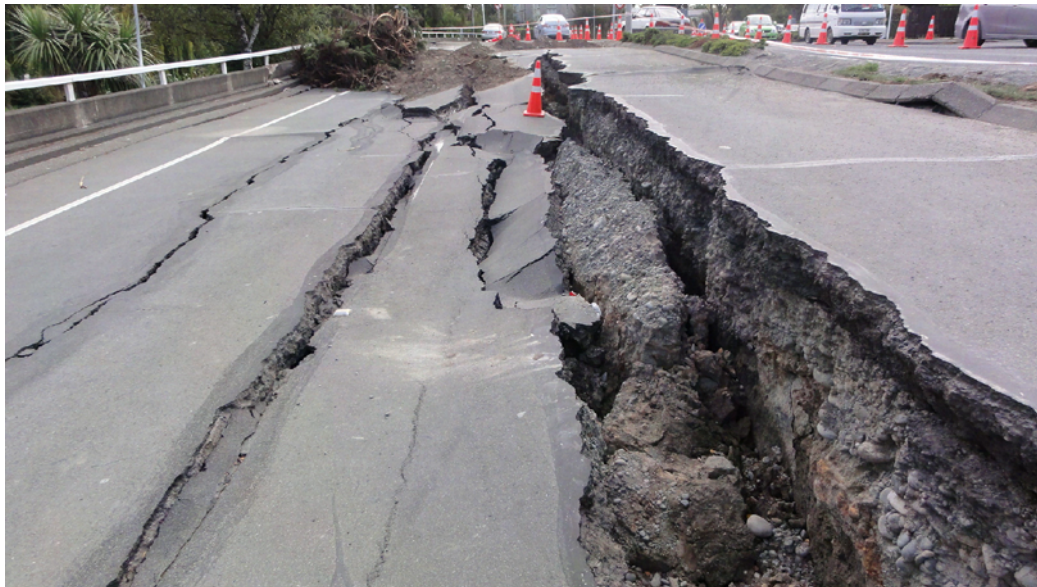
FAILURE OF ROAD DUE TO LIQUEFACTION AND LATERAL SPREADING IN THE 2011 CHRISTCHURCH EARTHQUAKE
