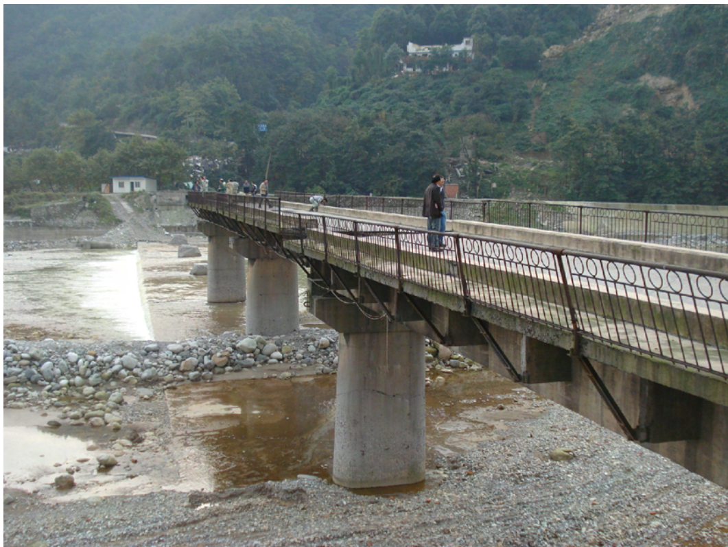
FAULT RUPTURE CAUSING BRIDGE COLLAPSE, ACCESS NOT RESTORED 6 MONTHS AFTER THE 2008 WENCHUAN EARTHQUAKE, CHINA
