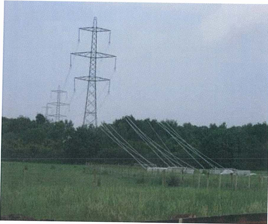
Photo 5: Conductors anchored to the ground at the end of wiring run
