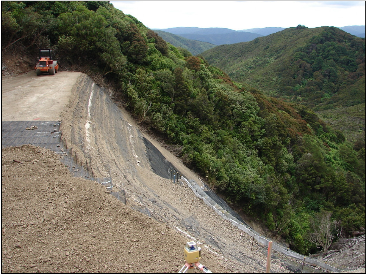
Figure 7.3: Example of a reinforced soil embankment under construction. Over time the slope face would be expected to re-vegetate
