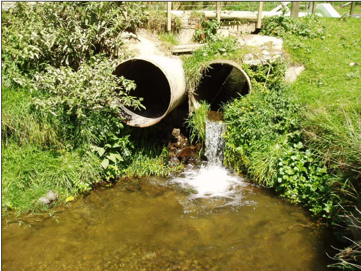
Figure 22.7: One of the existing perched culverts (acting as barriers to fish passage) in Duck Creek
