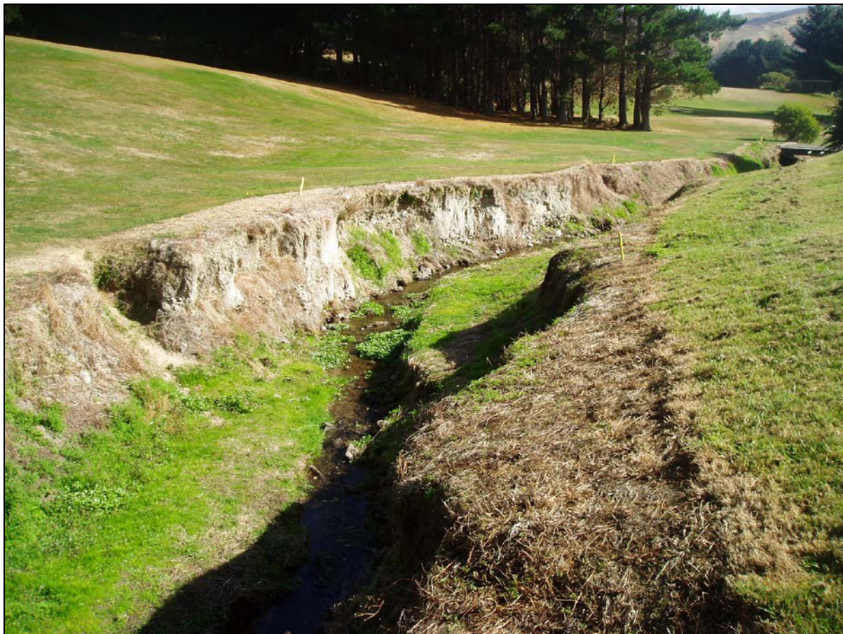
Figure 22.5: Mid Ration Stream with low flows and bank modification, running though the Pauatahanui golf course
