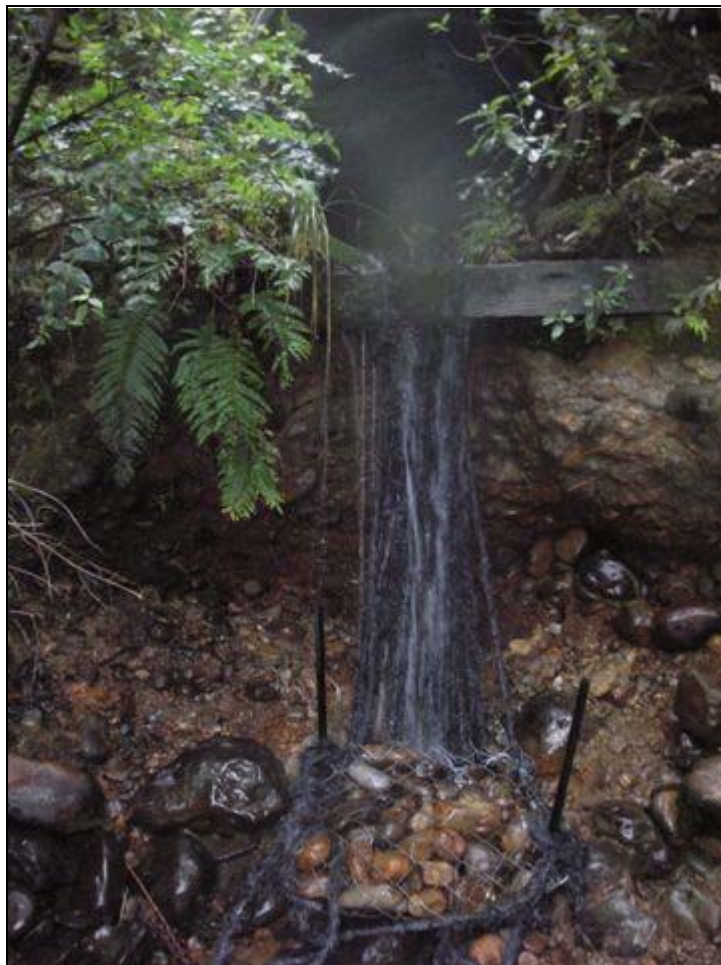
Figure 22.13: Example of a fish ladder
