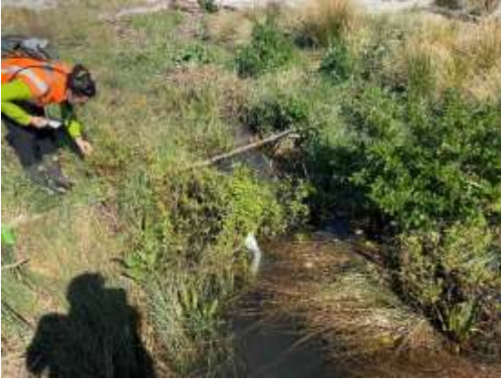
Figure 8 Culvert outlet from sea wall with deep pooling after rain.
