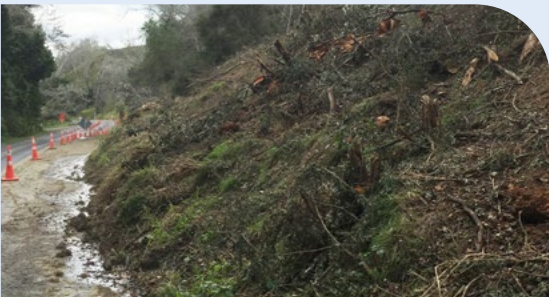
A slow moving slip on Otoko Hill - There is enough room here to build a temporary lane around the slip, creating two lanes and allowing contractors to clear and stabilise the site
