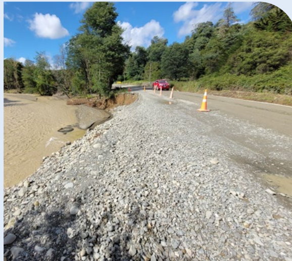
The washout at Makarika, north of Te Puia Springs, was temporarily repaired quickly by Blackbees
