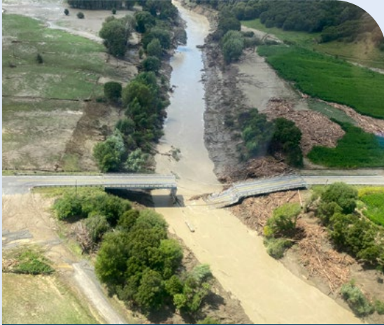
Hikuwai #1 Bridge was severed after Cyclone Gabrielle
