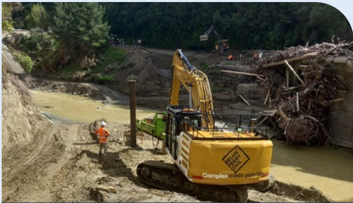
Contractors at work in the Waikare Gorge, where a Bailey bridge will be installed
