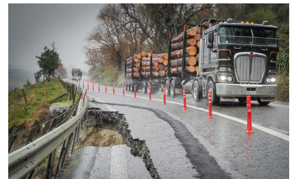
Slip on SH2 at Waikoau Hill
