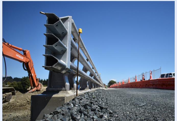
The safety barrier has been installed on the live lane side and will be installed on the opposite side once demolition of the existing bridge has been completed.
