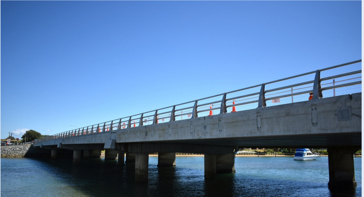
The new bridge from upstream site. The visible bolt holes are for a new architectural handrail that will help reflect the cultural importance of Taipa.
