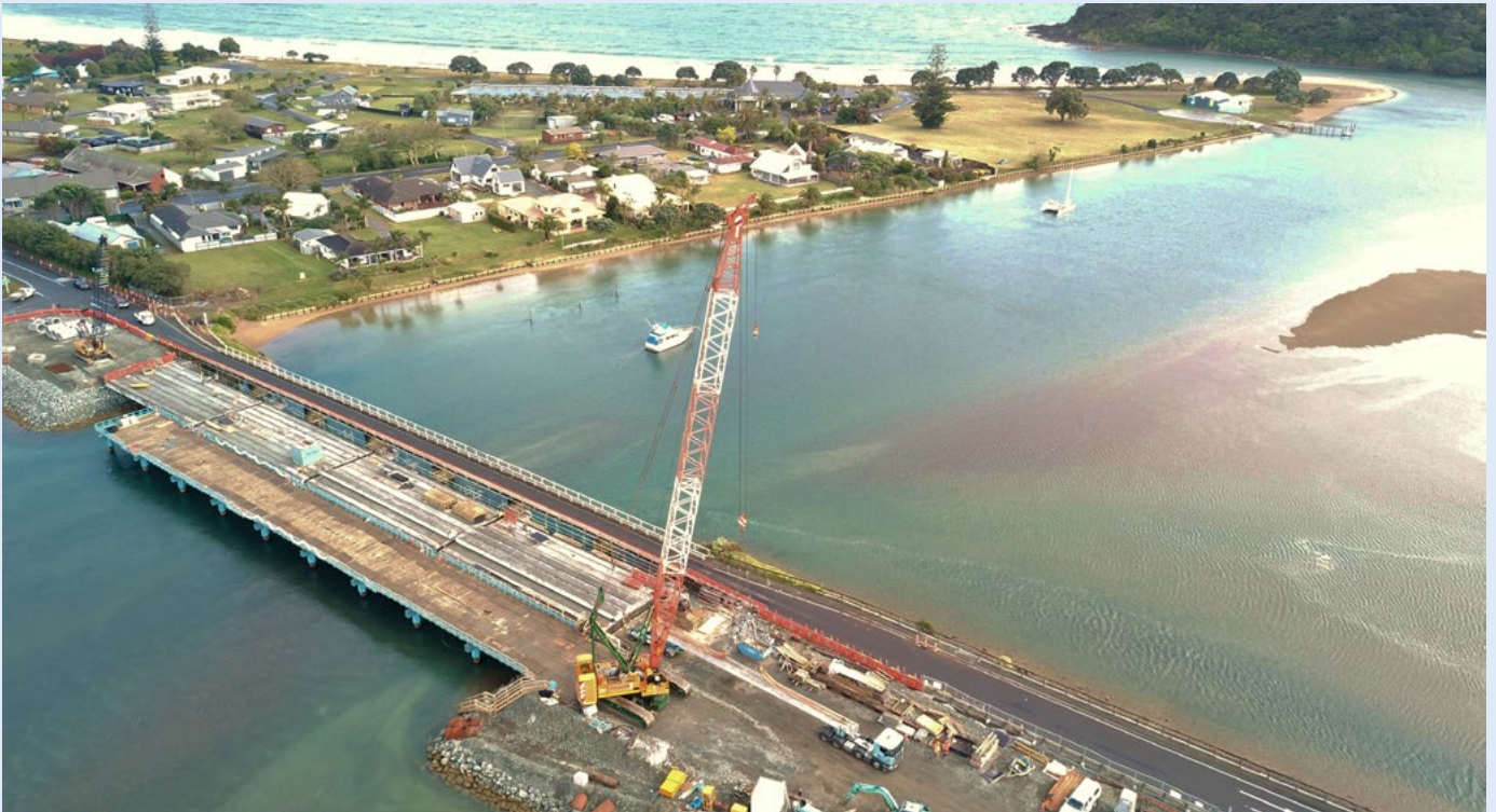
The bridge's four, 9 beam spans have been placed. Works will soon commence to remove the blue temporary bridge (staging).
